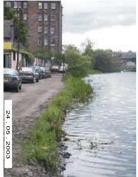
Plate 1. (below) A section of the original 1818 masonry revetment wall defines the present south bank. The garages on the left form the remnants of the late 19th / early 20th century brick buildings on Rope Walk.
