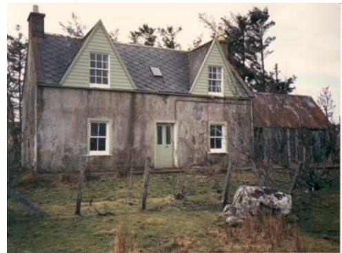
Croft 9's house before renovations took place - shoemaker's shed on the right
