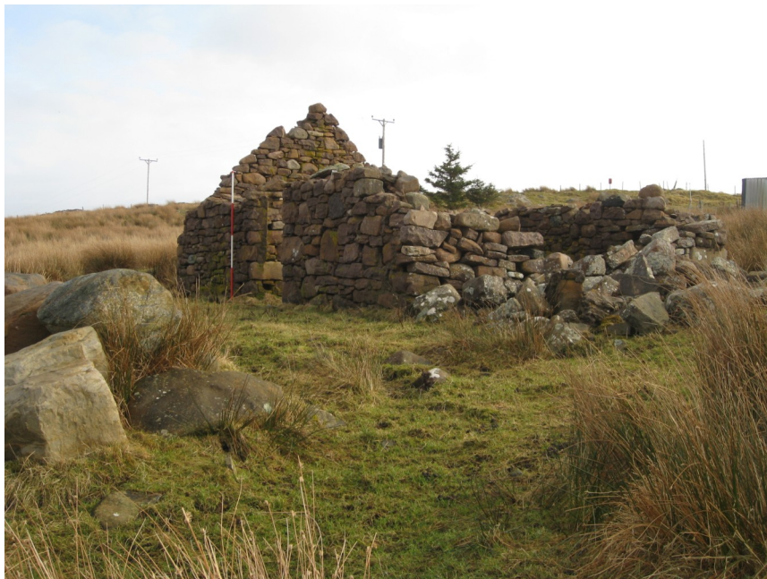
LOOKING SE AT COLLAPSED GABLE WALL AND RUIN
