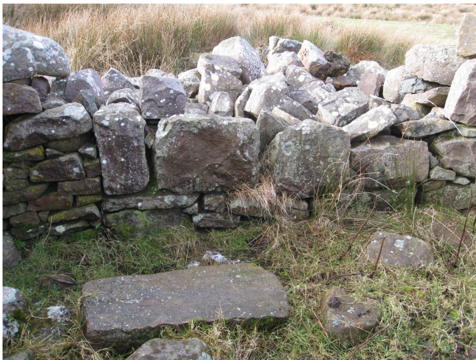
LOOKING W AT COLLAPSED INSERTED GABLE WALL
