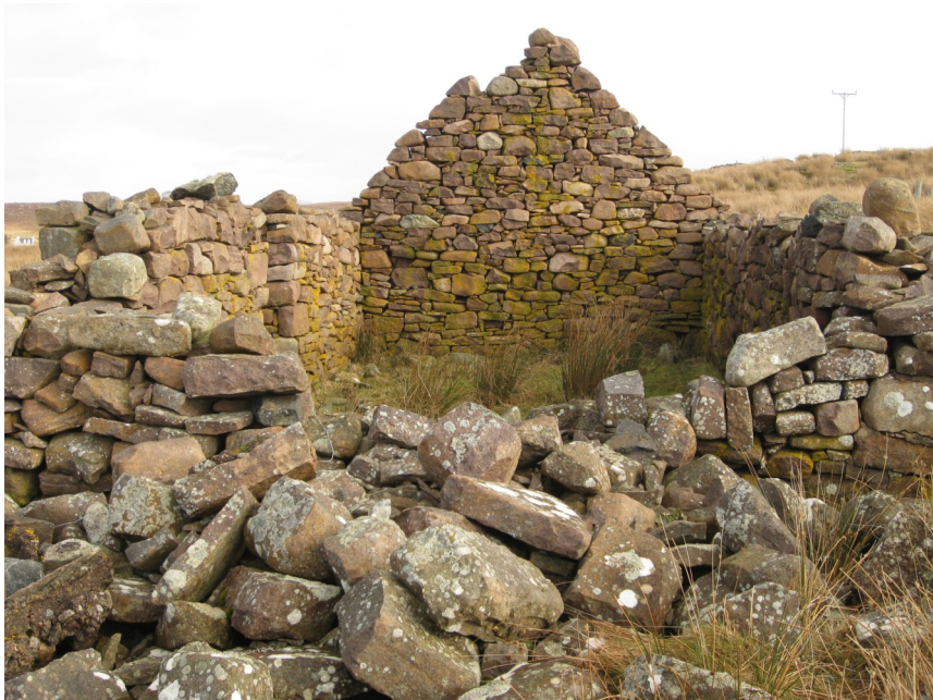
LOOKING E THROUGH COLLAPSED GABLE AT RUIN WALLS
