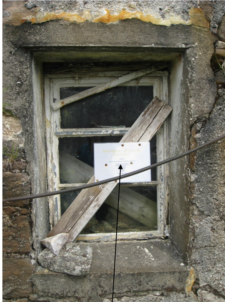
LOWER WINDOW BOARDED UP WITH NOTICE FROM HIGHLAND REGIONAL COUNCIL DECLARING HOUSE AS DANGEROUS.
