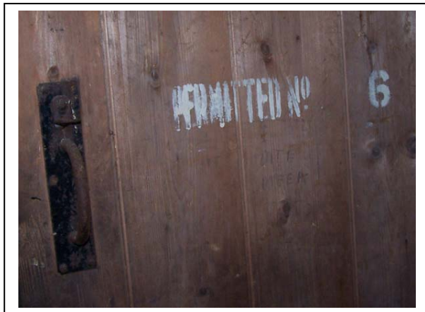
Figure 10 - Dormitory Door Sign – Occupancy (Peet 2011)
