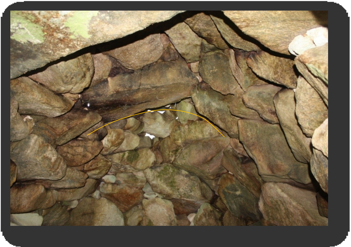
Figure 11 Taken looking up at the ceiling from the E, this image shows the highest part of the roof, formed by a combination of longitudinal and transverse slabs. Separated by the yellow line, the western end of the roof is formed by the continuation of corbelling from the end wall. 1148-355
