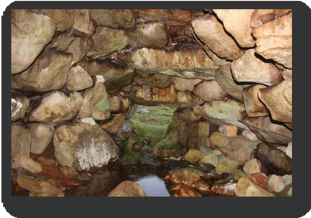
Figure 16 The brown silt fan at the bottom left of this picture shows where water is coming through the N wall from the ground beyond.
