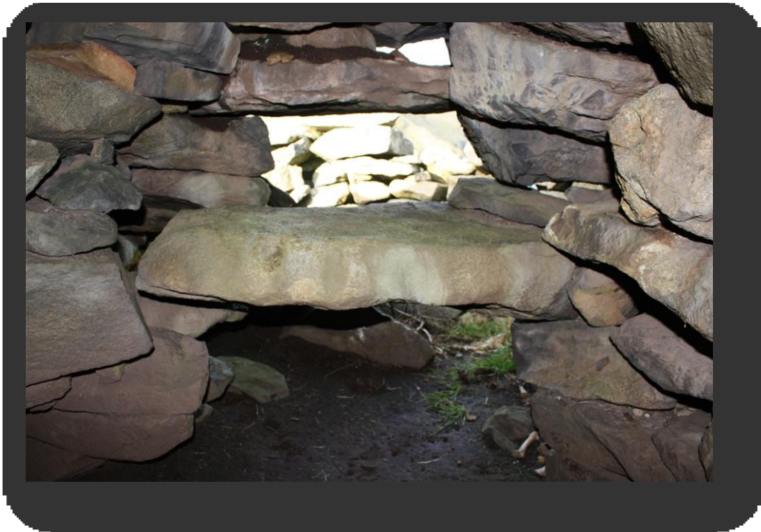
Figure 15 The lower lintel is not adequately supported on the left hand (S) side. Fortunately, it is not bearing a great deal of weight. 1148-103 © RCAHMS.
