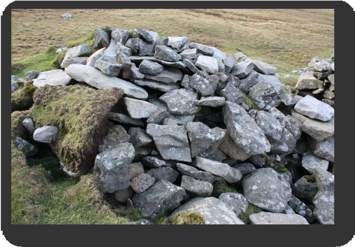
Figure 20 The large area between the SE and N cells that would benefit from a turf cap. 1148-120 © RCAHMS.
