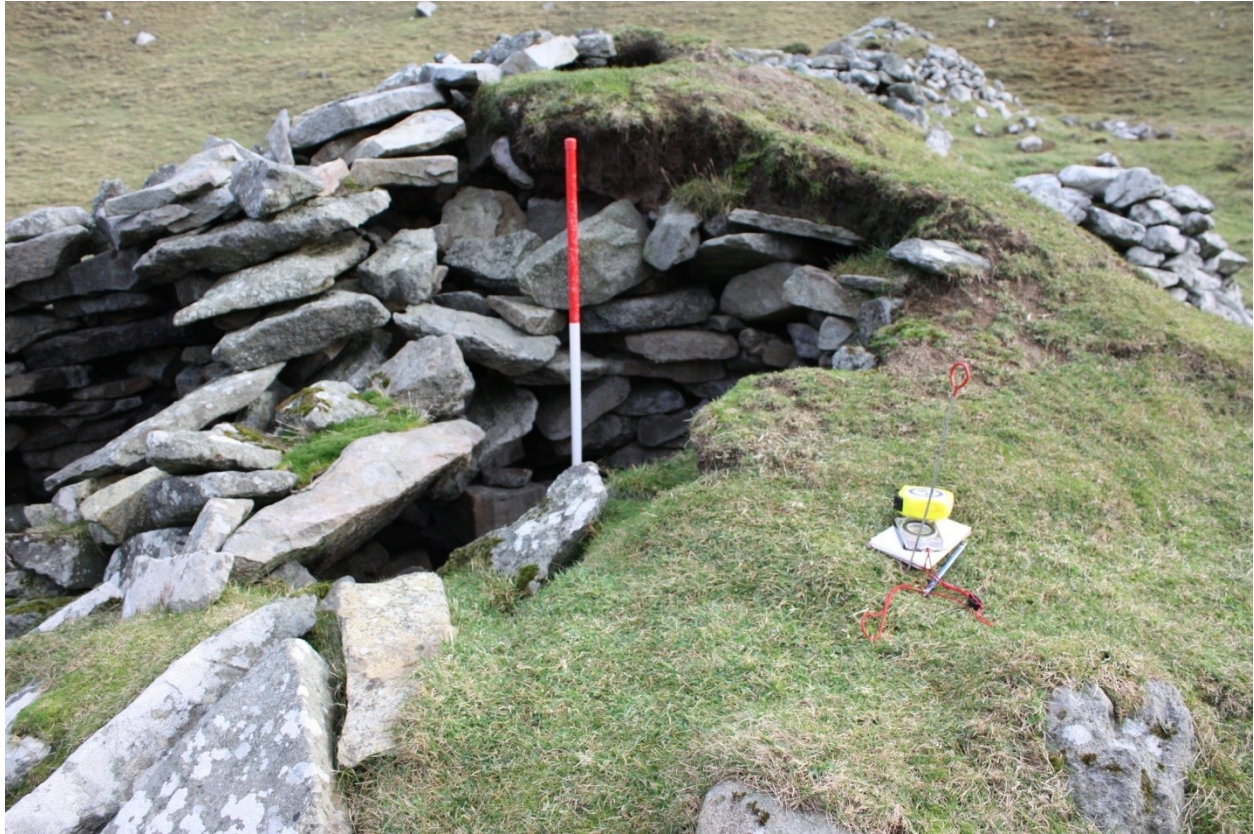
Figure 13 The S cell, in the centre of the picture, has collapsed. The masonry on the left of the picture is still actively collapsing, and it may pull the W wall of the roofed cell down with it. 1148-188© RCAHMS.
