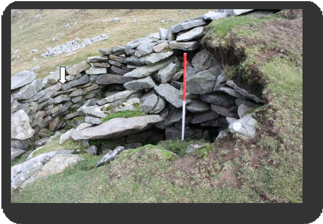
Figure 36 This image from 2010 demonstrates the level of collapse since the late 1950s. 1148-189 © RCAHMS
