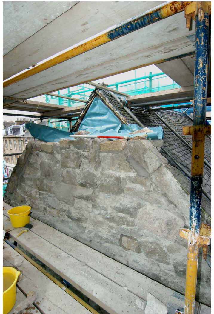
Plate 17 - Reconstruction of the gable apex following removal of the brick-built stack on the south-facing gable
