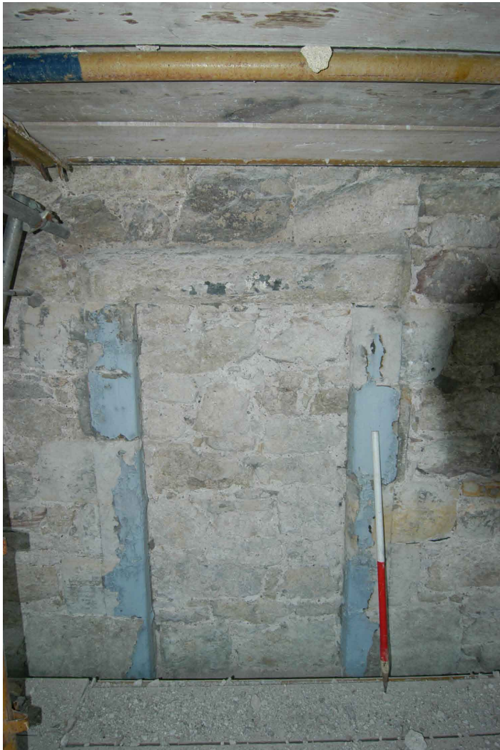
Plate 16 - The blind second-floor window on the south-facing gable following the removal of the harling
