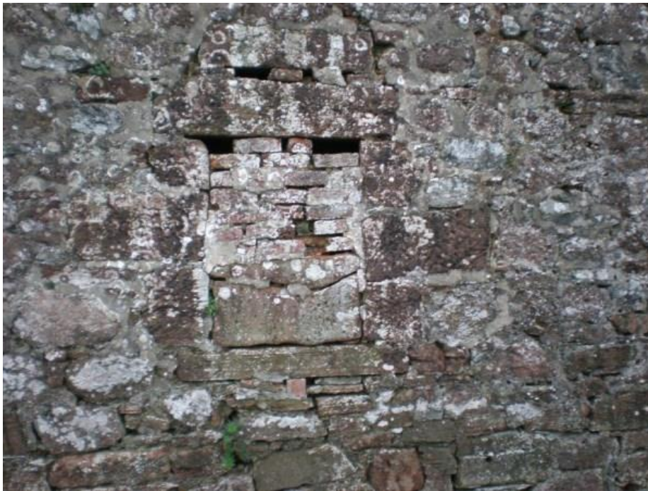
Blocked-up Bee Bole on North East Wall
