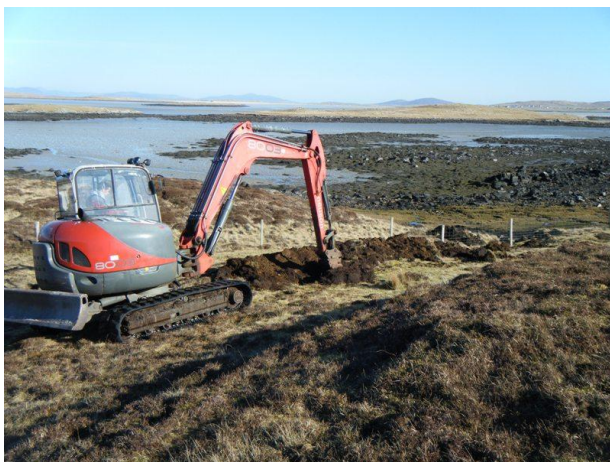
Illus 8: View of the excavation of the water pipe trench from the W.
