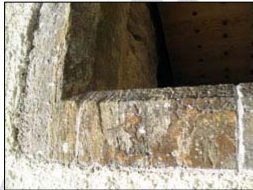
Fig. 2d: Detail of Quoins at Entrance
