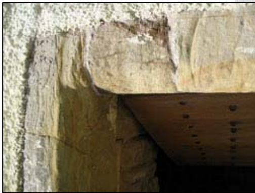
Fig. 2e: Entrance - Erosion at W side
