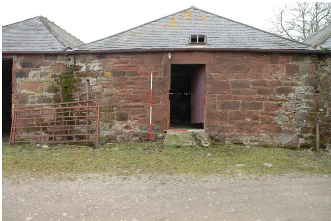
Illus 7 Steading wall 1 detail of change in wall construction ( to LHS of ranging rod)
