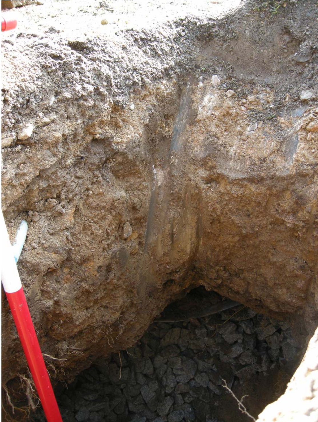
Illus 3 Soakaway in TP1
