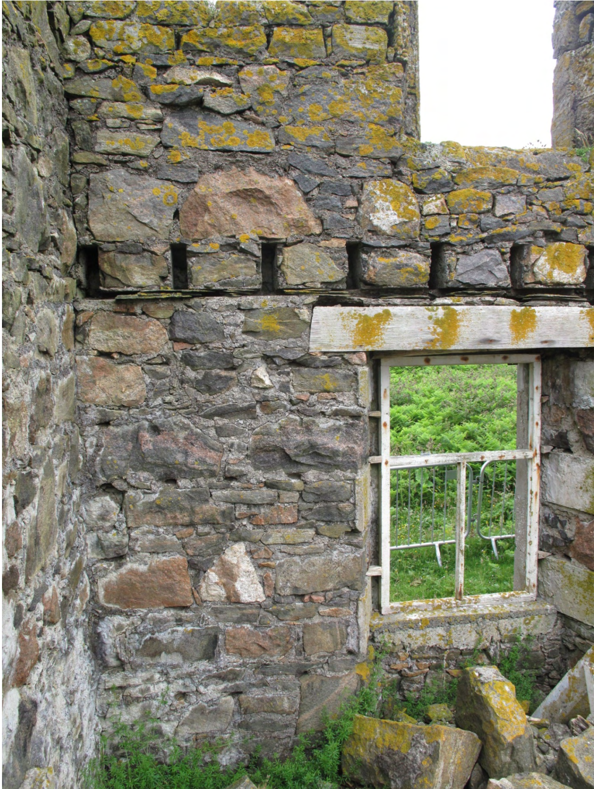
Figure 9 Nothing is left of the timber floor joists that were set in a leveling course of slates. The massive timber safe lintels are certainly of imported sawn softwood. The window frame is one of those put in during the 1970s restoration.
