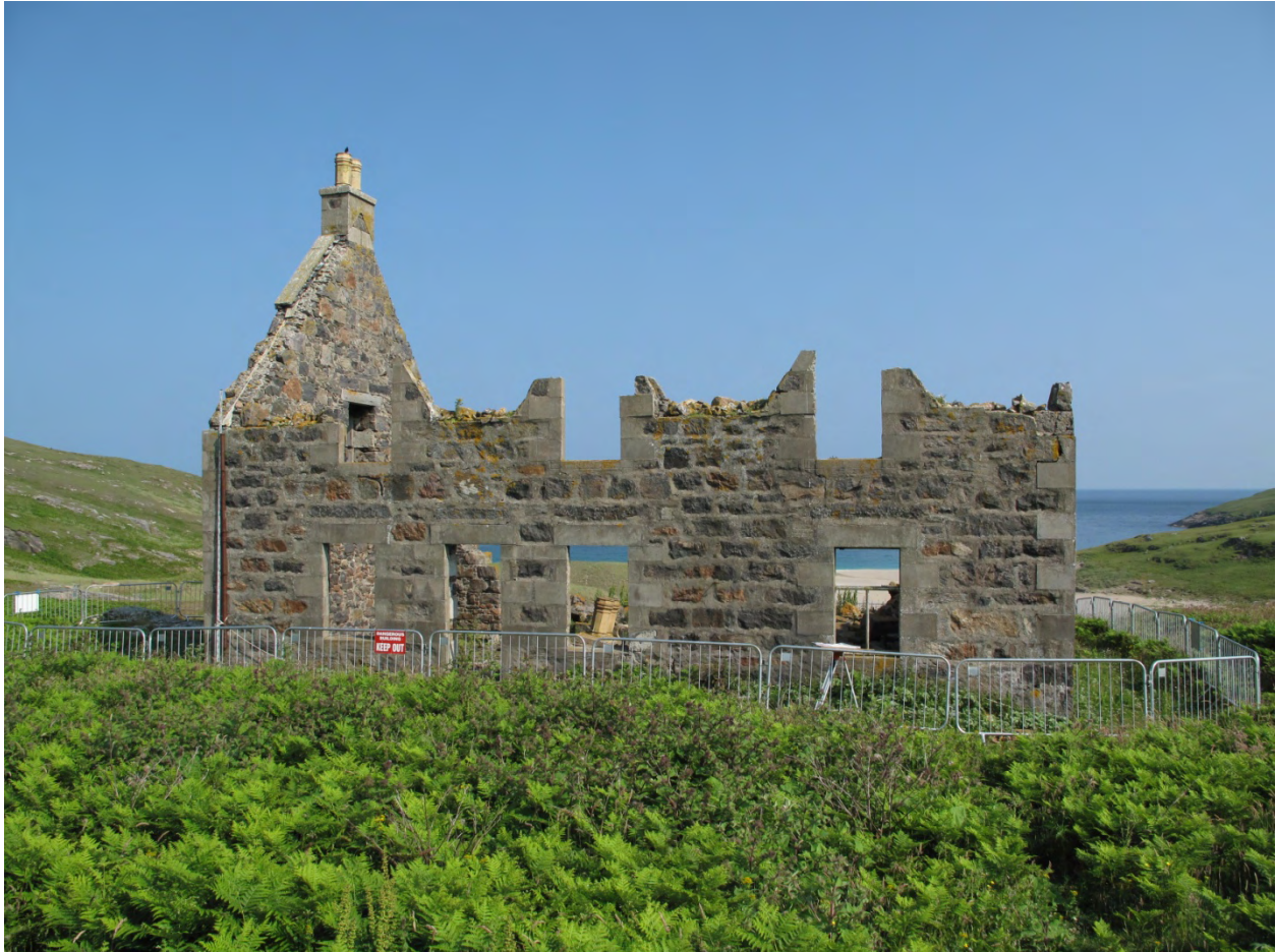
Figure 2 The back wall of the building is still straight, although the small stands of masonry that formed the half-dormers are coming away. Only one of the three drain-pipes is still in position, and much of the cast concrete coping to the gable has fallen off.
