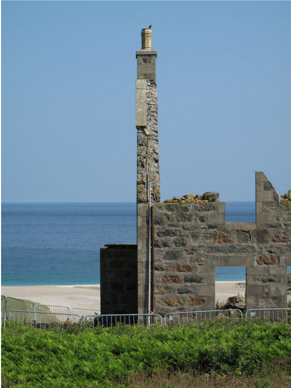
Figure 3 The gable can be seen in detail in this photograph. There is a final joist set into the gable to allow the sarking boards to be fixed to it. The sarking and the slate were tucked under the concrete coping, protecting them from the wind.
