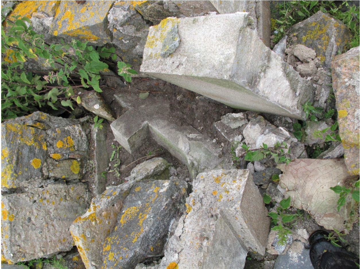
Figure 11 The concrete finial fell almost directly downwards from its original position, despite the fact that most of the front wall fell outwards. It was exposed for taking measurements, but left in situ.
