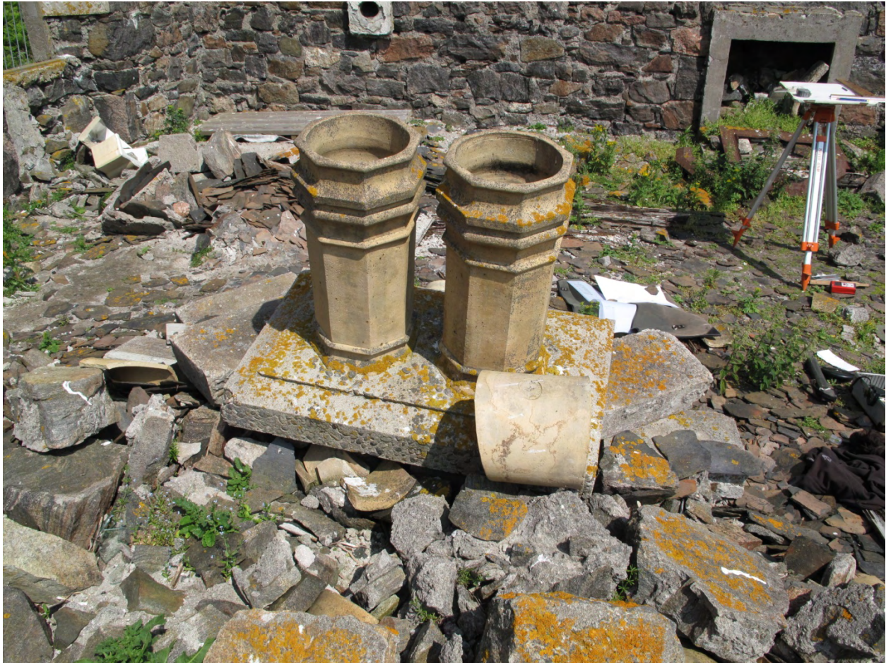
Figure 7 The floor of the building is strewn with collapse. The chimney cans survive, the whole SW gable having collapsed into the building. Beyond, there are slates, reddened by the recent fire, all over the floor. Fragments of the timber joists that held the floor can be seen, as can the flu of the kitchen stove and the fireplace.
