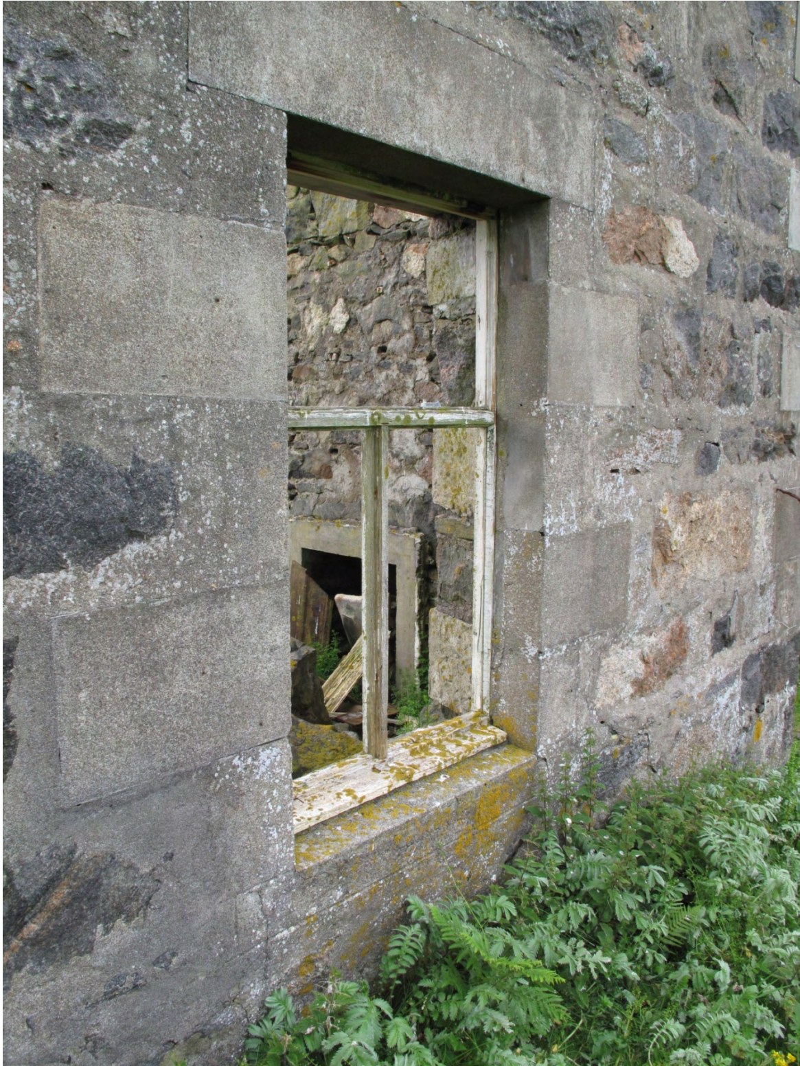
Figure 8 All of the openings are detailed with cast-concrete blocks. The windowsill has a slight fall to encourage water to drain away from the frame. The frame, which had a hopper window in the upper part, is from the 1970s.
