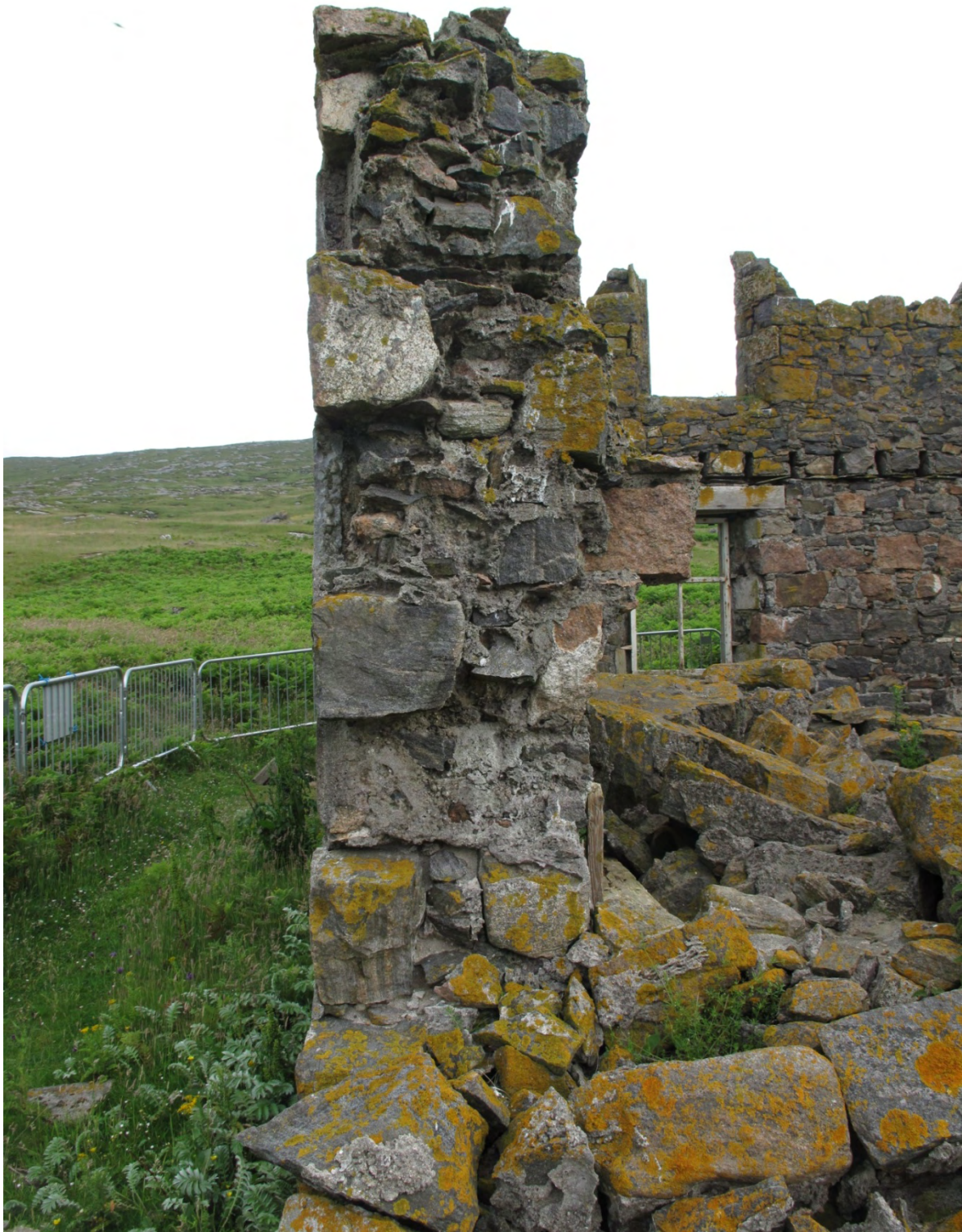
Figure 6 The wall is built with two faces of lime mortared stone, between which there is a filling of smaller stones and mortar. This section, where the concrete quoins have fallen away, one can see how the concrete was set against the wall-fill, and then a cement render was applied to the outside. The inside was lined with timber, held to the wall by timber dooks set into the wall.
