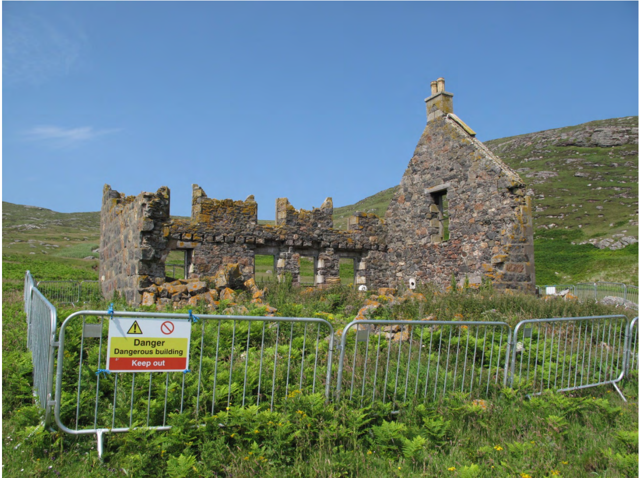
Figure 1 The ruinous chapel house from the south east. In part because of the way that the roof structure moved, bringing on the collapse of the structure, the gable has collapsed into the building, while the front wall has collapsed outwards. The remaining gable is still remarkably straight, as is the back wall.
