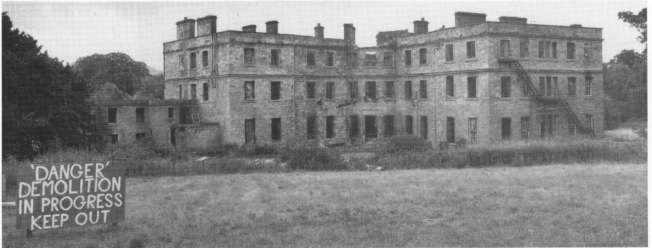
Minto House, Roxburgh District; general view from NE taken on the morning of demolition, 1 September 1992. [B74678]
