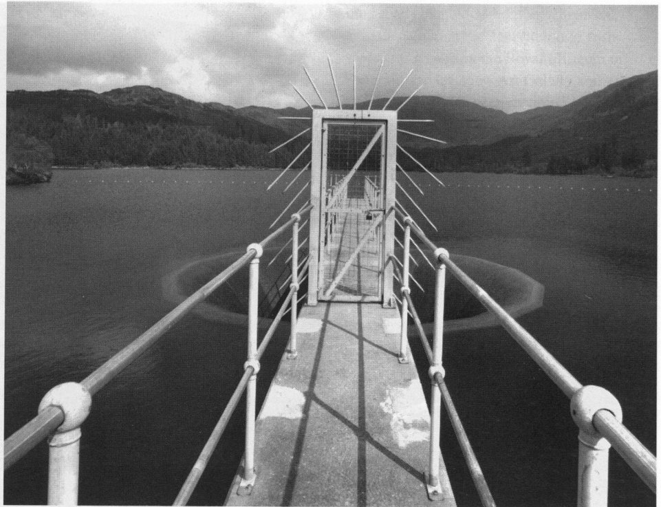
Barcaldine Alginate Works, Loch Creran, Argyll, reservoir in Gleann Dubh, entrance to spillway [C 68550]; settling tanks. [C 68515]
