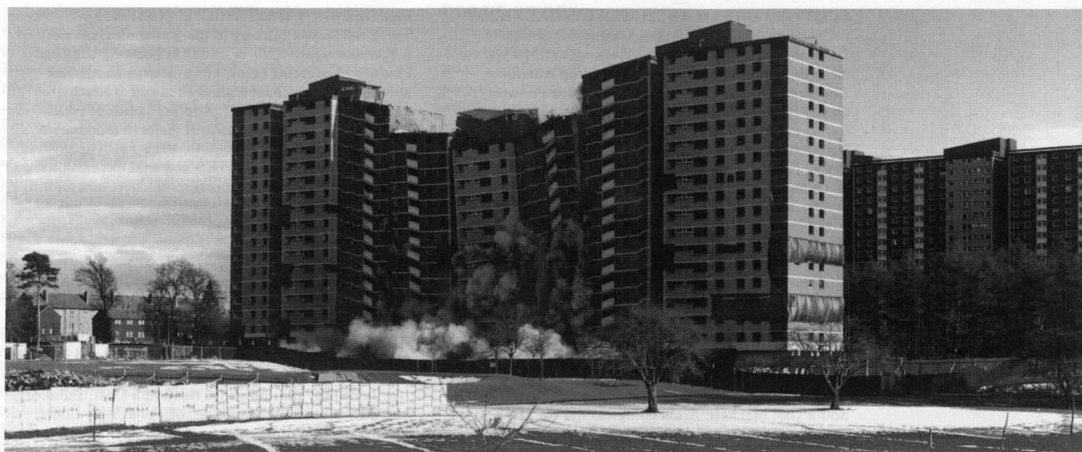
Demolition of a multi-storey block at Ardler, Dundee, February 1996. [C 65486 and C 65488]
