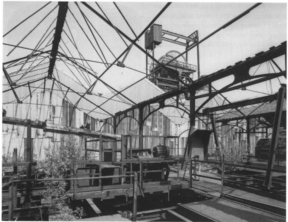
Lady Victoria Colliery, Newtongrange, Midlothian: view across upper level of pit-head complex, showing colliery headgear in background. [D28555]
