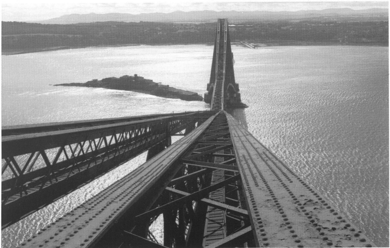
Plate 4: View from north (on top of Fife erection) of south parts of the Forth Bridge (B 3219, 1988, RCAHMS, item 121).
