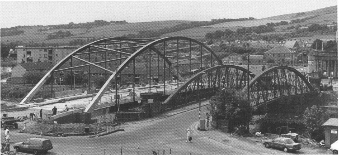
Plate 8: View from north-east of the new Bonhill Bridge under construction, with the old bridge also visible (right) (B 13300, 1987, RCAHMS, item 17).
