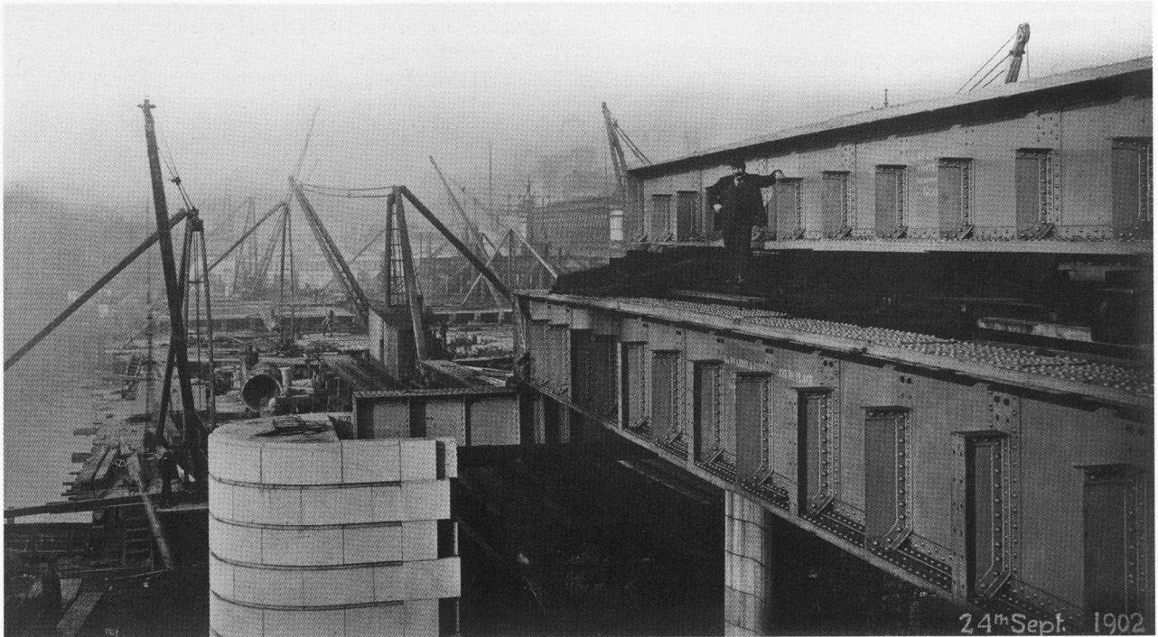
Plate 13: View from Clyde Place, Glasgow, of the Central Station Bridge during construction, September 1902 (completed 1905). This was built for the Caledonian Railway Company to their design as part of the reconstruction of the station. An earlier bridge built also by Arrol (1875-8) for the Caledonian Railway is just visible in the centre background. Its girders and decking had to be jacked up by 3 feet in order to achieve the rail level of the new bridge (B 91884 PO, item 58).
