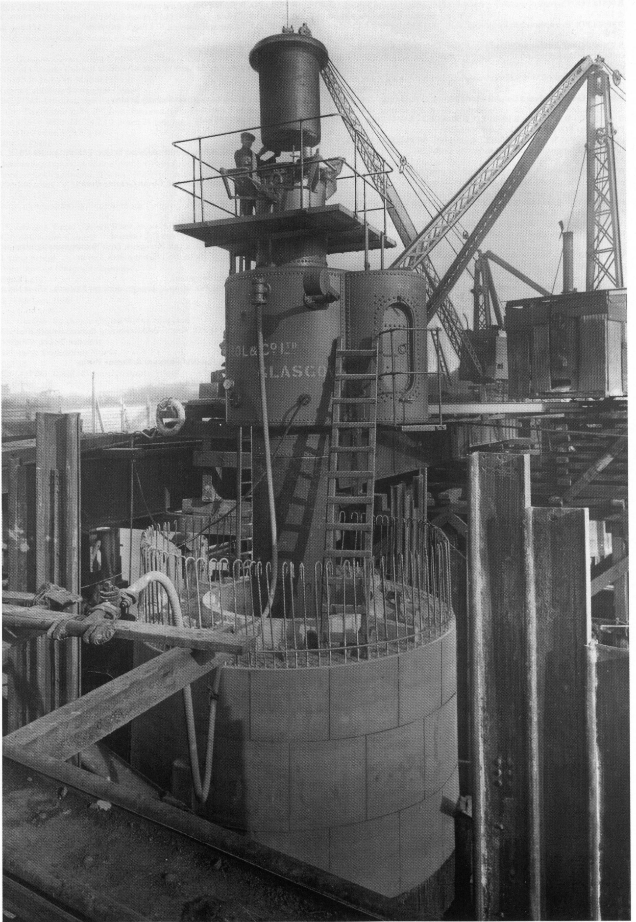
Plate 17: View of King's Road Bridge, Ballater Street, Glasgow, showing the existing bridge to the right and the air lock used for excavation of pier foundations, 1931 (B93328 PO, item 69).
