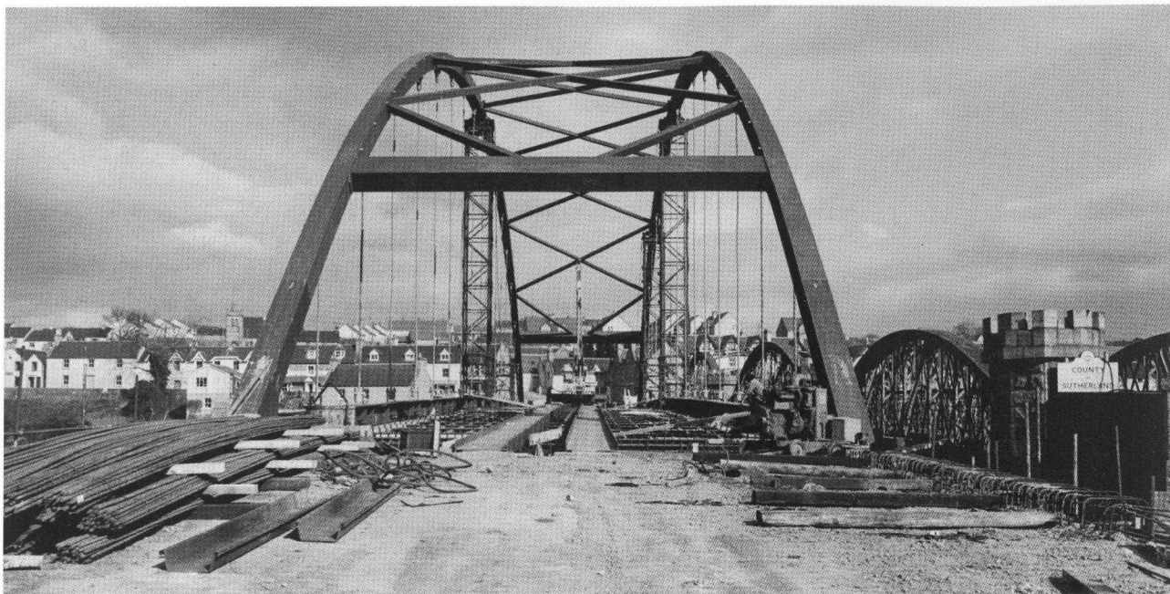
Plate 21: The elegant bow-string girder (new) Bonar Bridge under construction, viewed from the west abutment in March 1973. This was built to replace an earlier Arrol braced bow-string girder bridge of 1894 (C 87954 PO, item 107).
