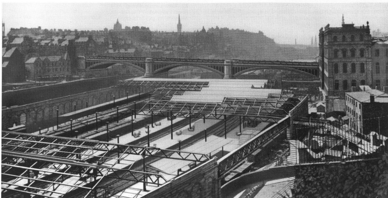
Plate 19: General view (enhanced for publication) of Waverley Station and the North Bridge, Edinburgh c.1908. Sir William Arrol and Company carried out the work on the North Bridge to a design by Blyth and Westland of Edinburgh. This is possibly the original publication photograph used in Bridges, Structural Steel Work and Mechanical Engineering Productions , 1909, 123-5 (B 93379 PO, item 85).
