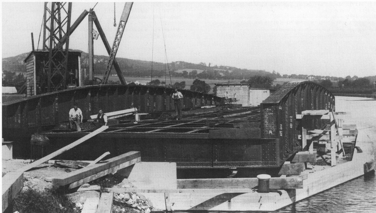
Plate 12: View of the replacement Tomnahurich swing bridge under construction over the Caledonian Canal, 1938 (B 91719 PO, item 38).
