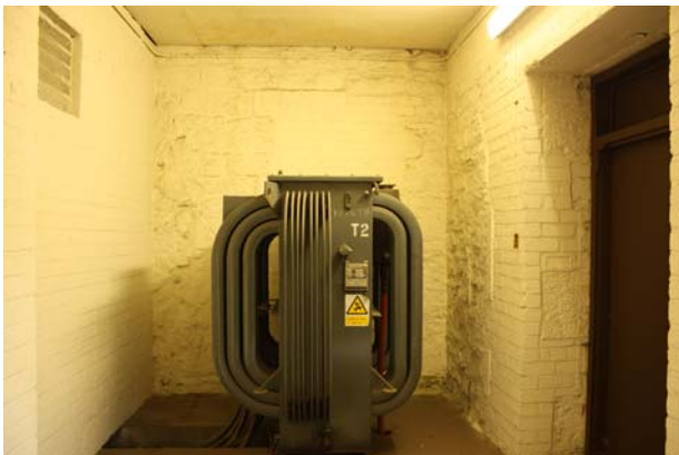
Illus 20: Eastern guardhouse, Transformer 2 in Room 2
