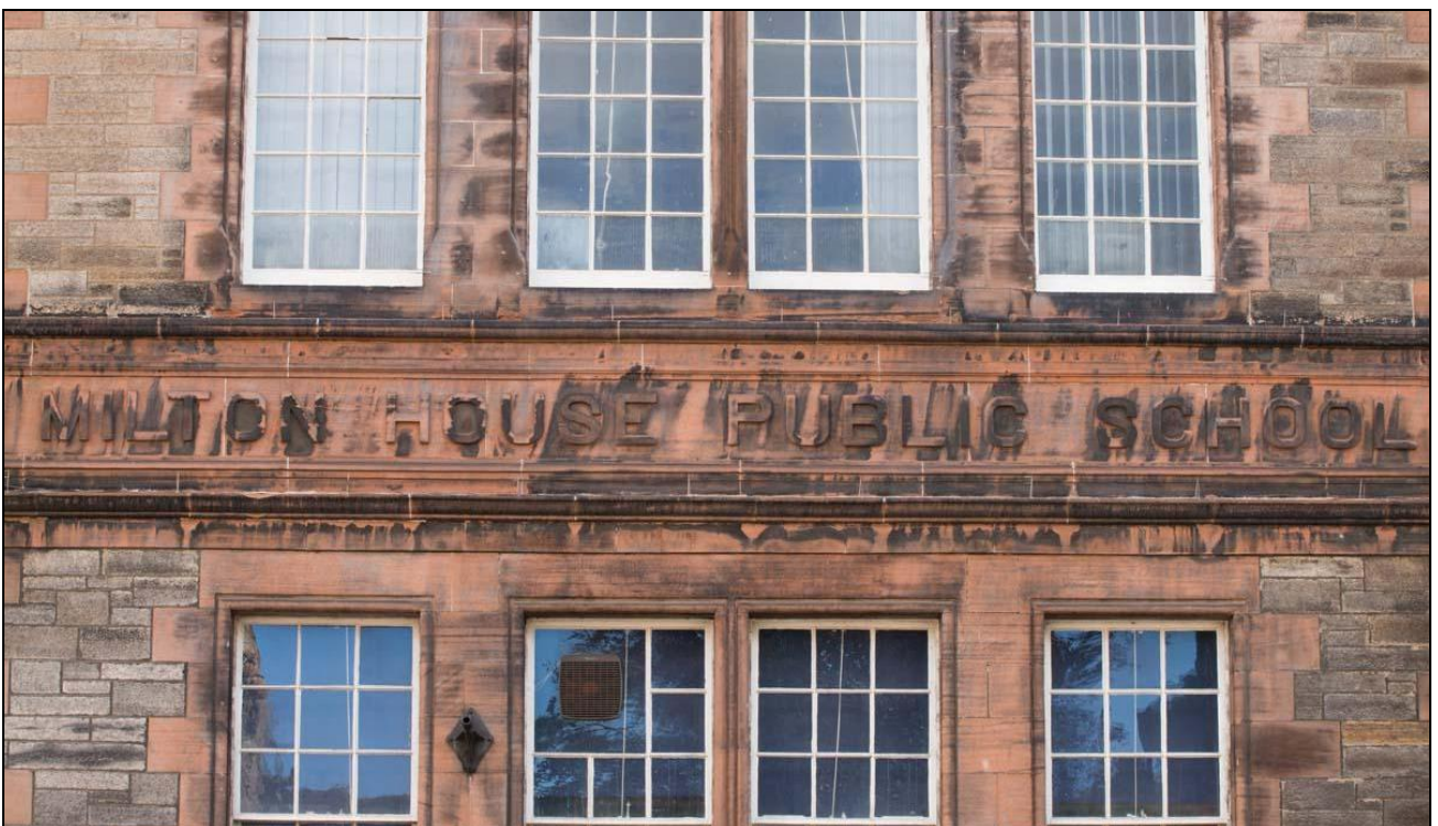
Figure 15: Detail of carved stonework on front elevation of Royal Mile Primary School (formerly Milton House Public School), 2014 (DP161366 ©Crown copyright HES)
