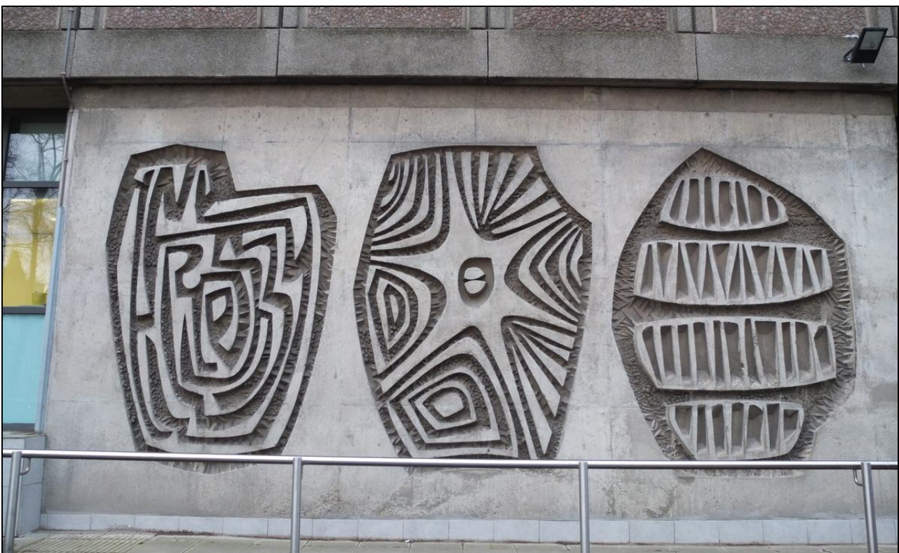
Figure 202: Detail of three of four sculptured stones at entrance to Charteris Land , St John Street, 2015 (DP205187 ©Crown copyright HES)
