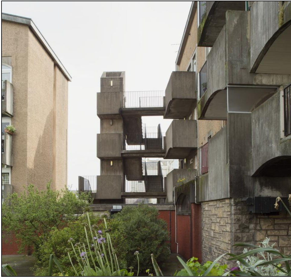
Figure 171: View of stairway to rear of 1-3 Brown's Close/65-71 Canongate, 2014 (DP188682 ©Crown copyright HES)
