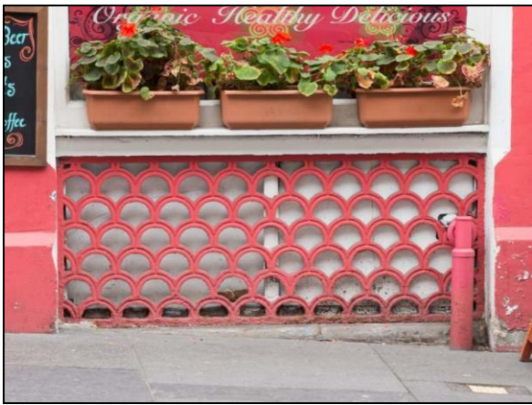
Figure 49: Detail of decorative grille below shop window at 6-8 St Mary's Street , 2013 (DP161645 ©Crown copyright HES)
