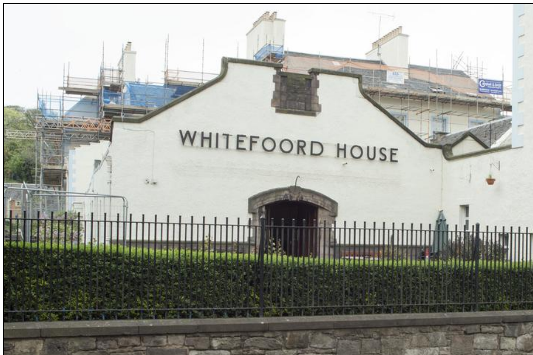
Figure 144: View of former poppy factory at Whiteford House , from south, 2014 (DP190206 ©Crown copyright HES)
