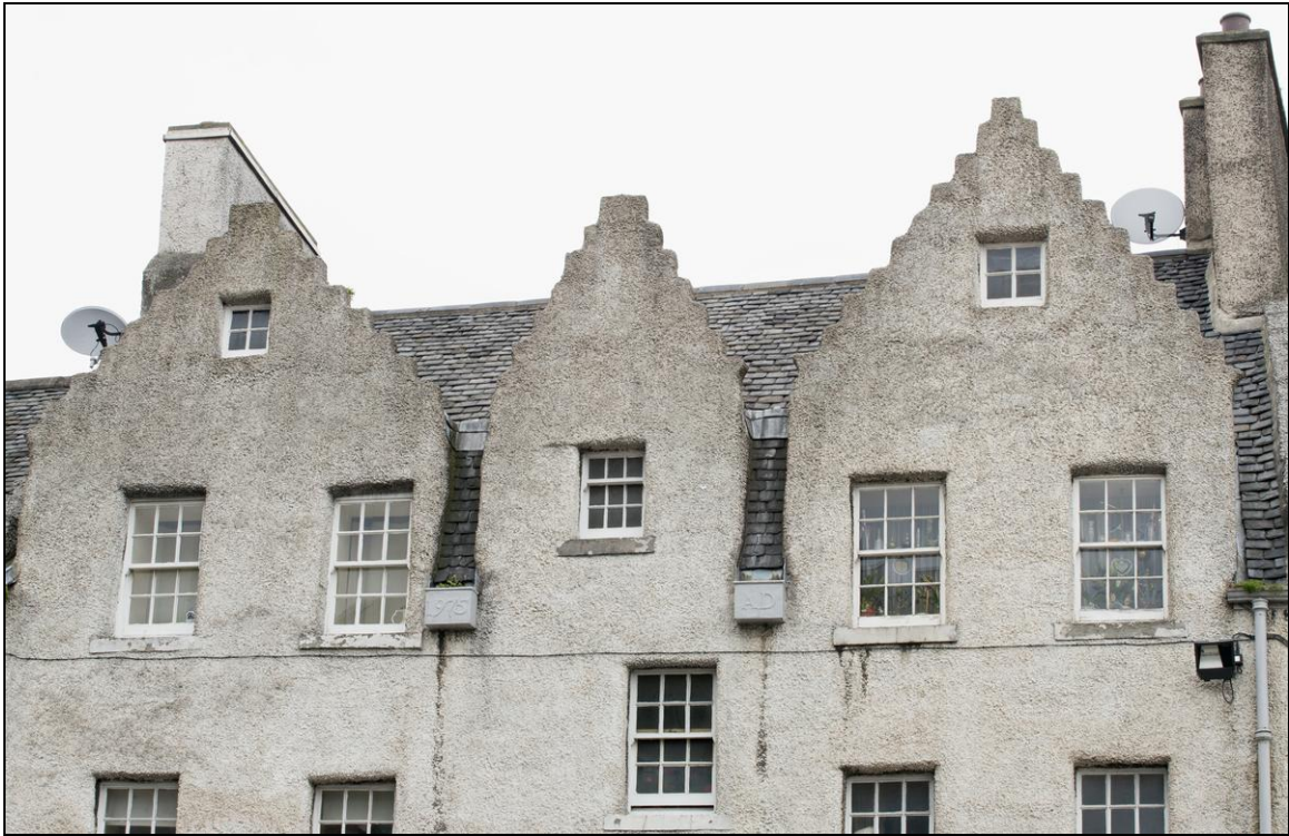
Figure 174: Detail of crowstepped gables on front elevation of 5 Canongate , 2014 (DP188699 ©Crown copyright HES)
