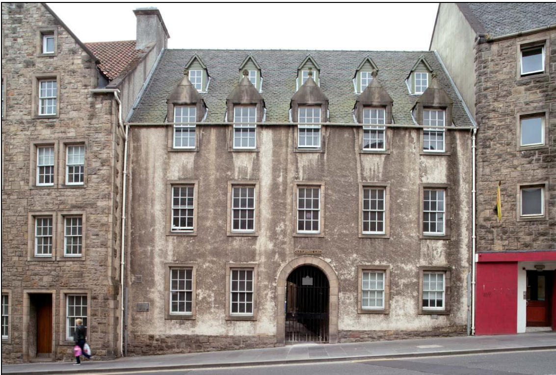
Figure 159: View of Playhouse Close and Old Playhouse Close at 194-200 Canongate, from north, 2013 (DP160529 ©Crown copyright HES)
