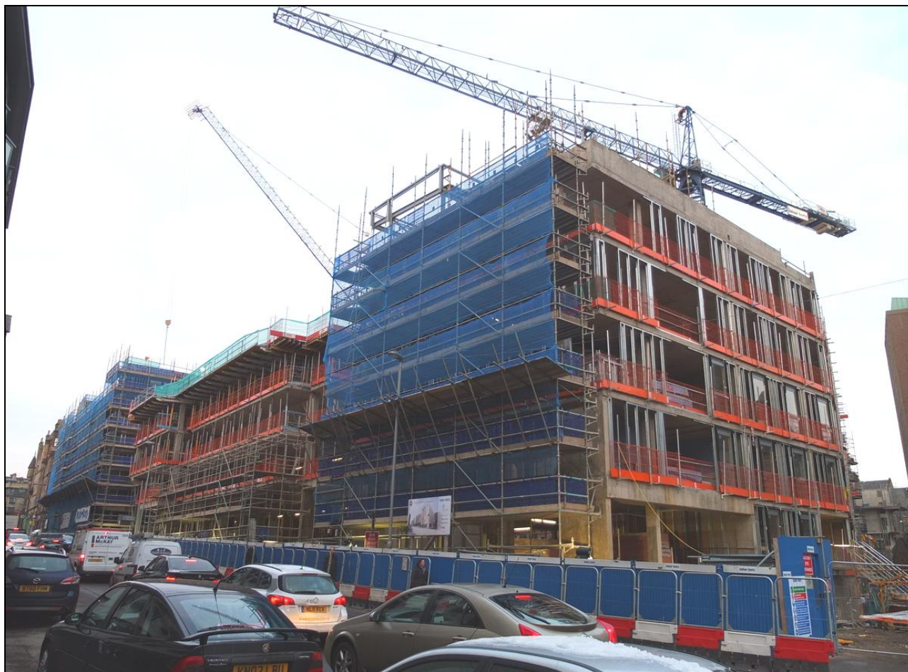
Figure 213: View of University of Edinburgh student accommodation under construction at Holyrood Road, from east, 2015 (DP205189 ©Crown copyright HES)
