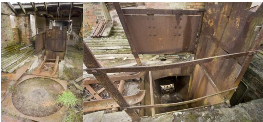
Above left: View from west of tipping area for tub into crusher for Pan Mill below [DP111682]. This has been inserted into an existing floor. Above right: Detail of tipping area with crusher jaws visible on frame below from south. The Pan Mill is directly beneath the camera [DP111681]
