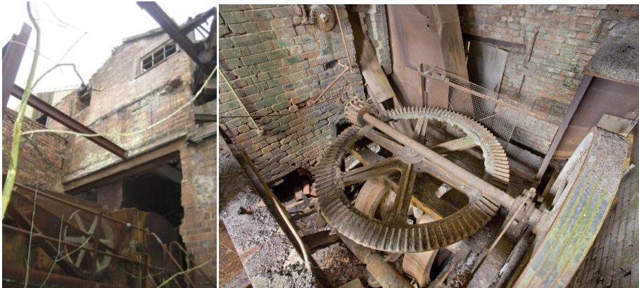
Above left: Old Pan House. The slapped through wall clearly is visible and the steel structure carrying the crusher which fed the Incla Mill. The gable above is clearly later (possibly the 1930s). Image: M McDonald, 2011
