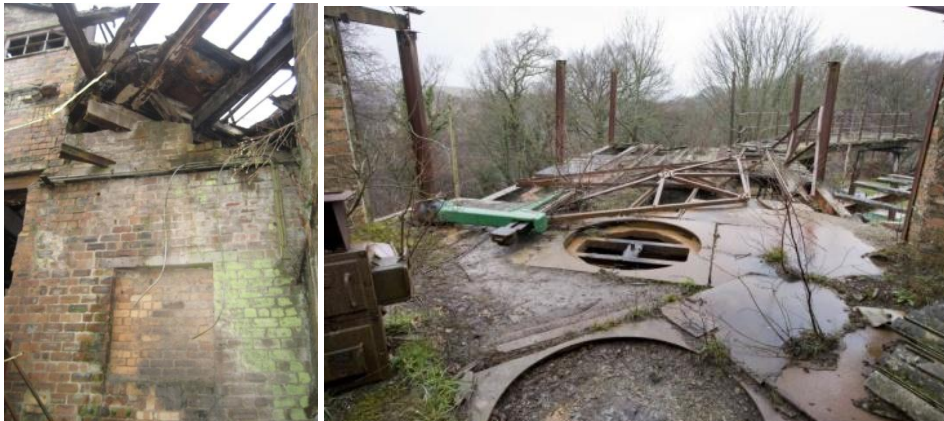
Above left: South wall of Old Pan House (Building showing blocked doorway to Haulage Building (Building B) and the insertion of the incline above. The slatted through wall of A2 (to insert crusher and motor gantry) visible on left. Image: M McDonald, 2011 Above right: Clay distribution Top of incline with turntable (gone) scales for weighing full tubs, tub backing up area and run of mine rails (extreme right). RCAHMS, 2011 [DP111683].
