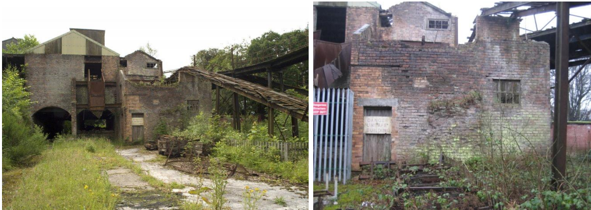
Left: North end processing buildings, original c.1916 (and modified) Old Pan House, incline and 'run of mine' incline on right, with chute on left. Double arch area is the undercroft of the hopper area may also date from c.1916, although modified and extended at the south end post -1946. RCAHMS, 2011 [DP028266]. Right: East elevation of the Old Pan House (see SC SC1361815, A) remodelled to accommodate the later hopper area (just visible, left). The 'run of mine' rails on right are precariously balanced on a brick pier on the wallhead. This building was still roofed until at least the closure of the site in 1980 1946. Image: Miriam McDonald, 2011.
