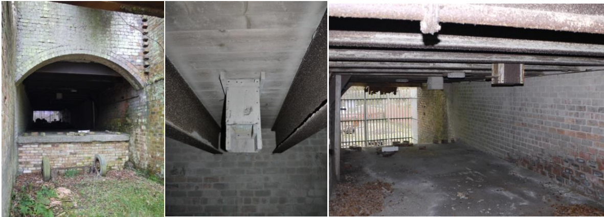
Above left: View of Loading Bay below Hopper C from south. This was originally served by railway wagons but was converted to allow bagging and loading into lorries. Image: M McDonald, 2012 Above centre: Funnel from modified hopper above to allow bag filling. The bags were then manhandled into the bag sewing area and loaded onto lorries. Above right: View from north of platform and funnel for filling bags with dry clay dust from modified hopper floor above. Image: M McDonald, 2011
