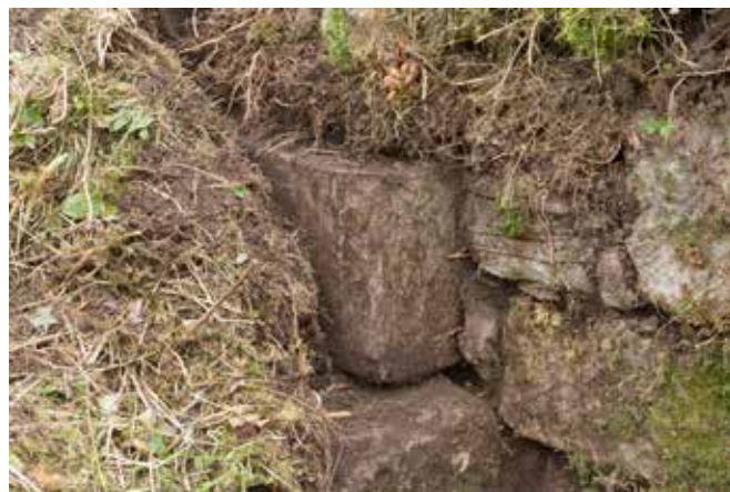
Fig 22 Arrow-shaped stop at the base of the chamfered stonework of the entrance opening. DP151880
