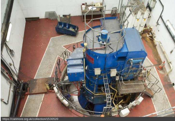
Circulating Water Pump House. CW Pump 1. Seawater was taken in through fixed bar, removable smolt and maintenance screens to remove debris. The water then went through the intake tunnel and through drum screen to the pumps. [DP 237603, 2016. Crown copyright: HES]
