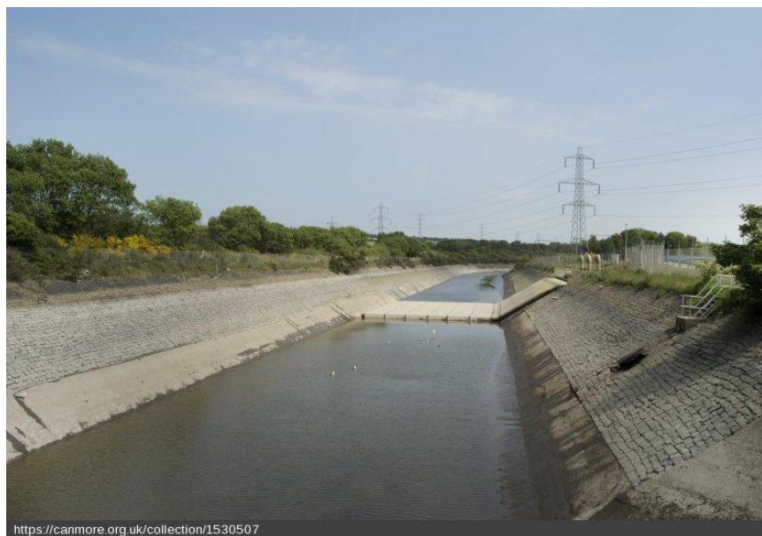
https://canmore.org.uk/collection/1530507 General view of water cooling channel or flume outflow from south west. [DP 237519, 2016. Crown copyright: HES]
