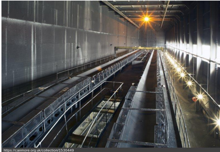
Interior general view. Boiler House. Ground floor level (44 feet level). Shuttle conveyor no. 25 and 26 - system of delivering coal (via 31 conveyors in total) to boiler units [DP 237532, 2016. Crown copyright: HES]
