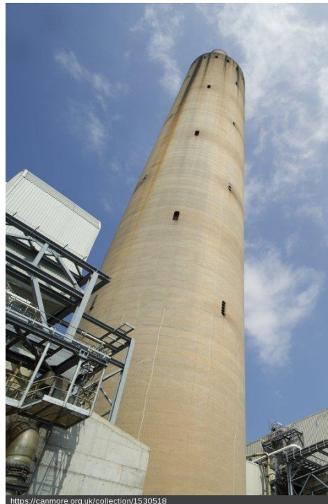
The Longannet 183m high chimney with its concrete windshield protecting the four flues. [DP 237601, 2016. Crown copyright: HES]
