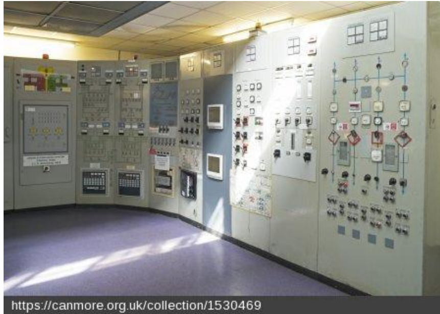
https://canmore.org.uk/collection/1530469 Central control room, annex. Part of switchhouse control panel. [DP 237552, 2016. Crown copyright: HES]
