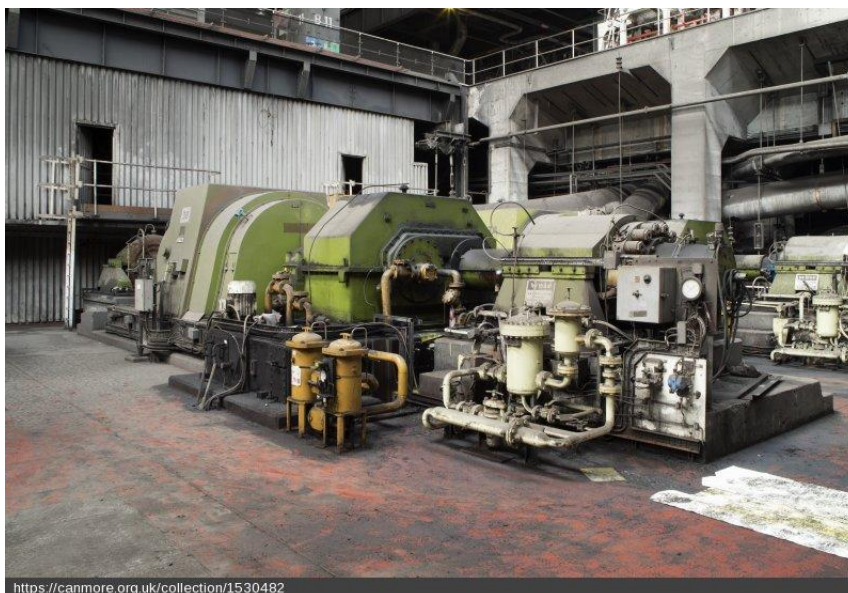
https://canmore.org.uk/collection/1530482 Turbine Hall. Boiler feed pump. G and J Weir Ltd. [DP 237565, 2016. Crown copyright: HES]
