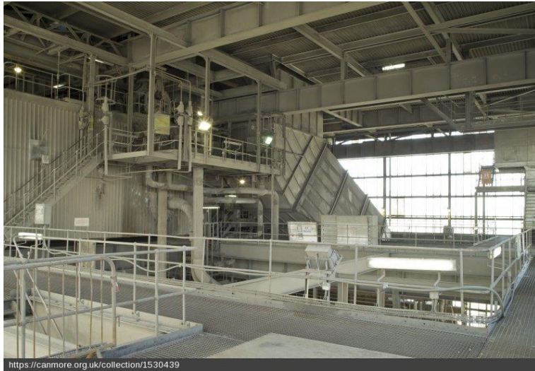
Boiler House (198 foot level) Unit 4 boiler forced draught fan suction inlet duct. [DP 237522, 2016. Crown copyright: HES]
