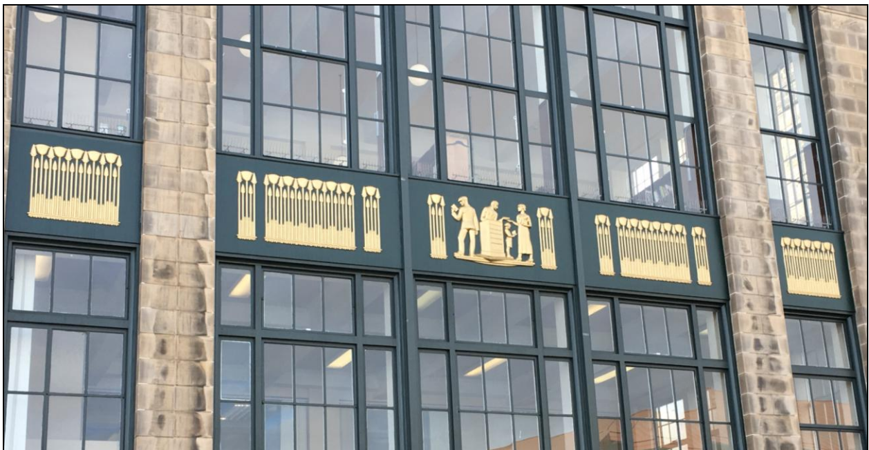
Figure 148: Detail of painted bronze-plated cast-iron panels on Dundee Street elevation of Fountainbridge Public Library, 2017 (DP260083 ©Crown copyright HES)
