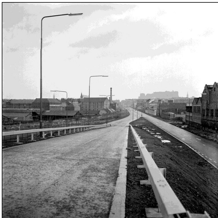
Figure 13: View of West Approach Road on the day it opened, December 1974 (©The Scotsman, copied from SCRAN: http://www.scran.ac.uk/database/image.php?usi=000-000-541-602-R&csi=000-000-541-602-C&scache=3db7adnmk0&searchdb=scan )
