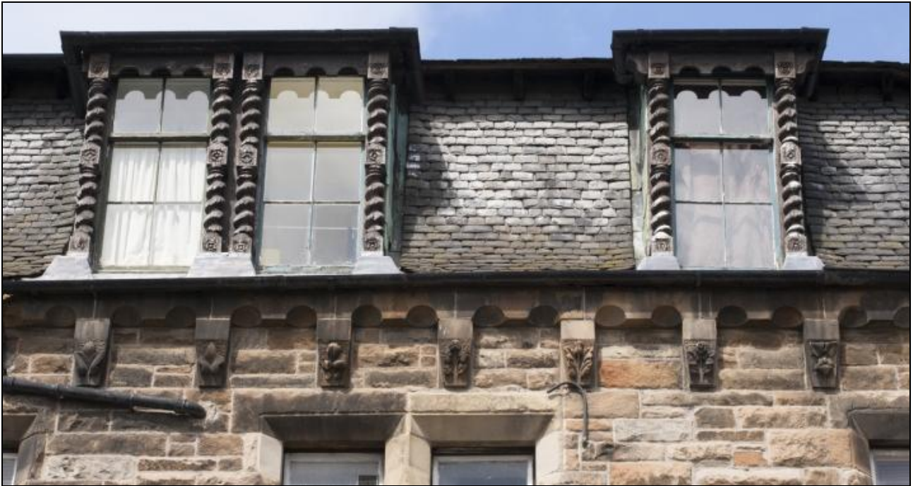
Figure 100: Detail of carved mullions and corbels at attic level of 158-164 Fountainbridge, 2014 (DP203634 ©Crown copyright HES)
