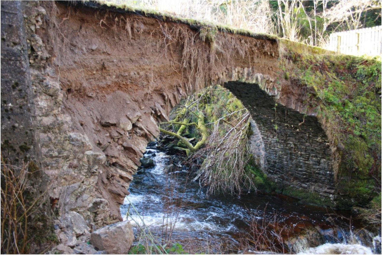
Plate 3: Detail of the recent collapse of the bridge.
