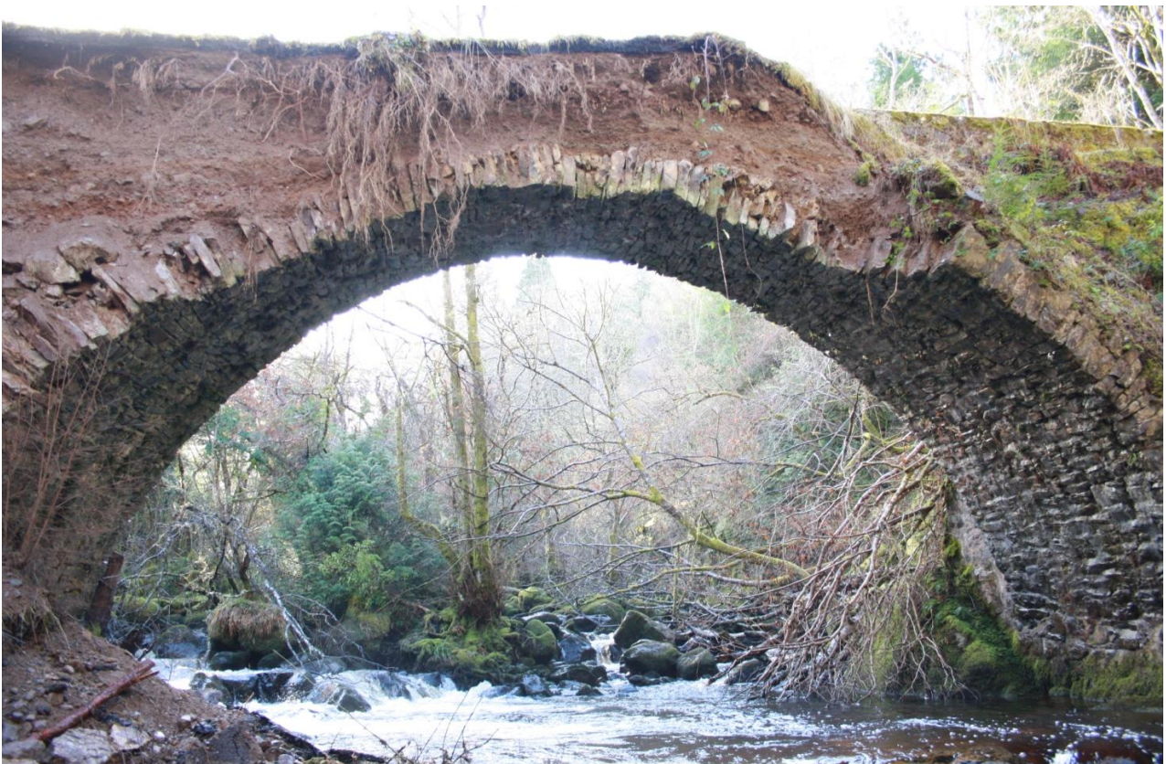
Plate 4: View of the recent collapse from the W.
