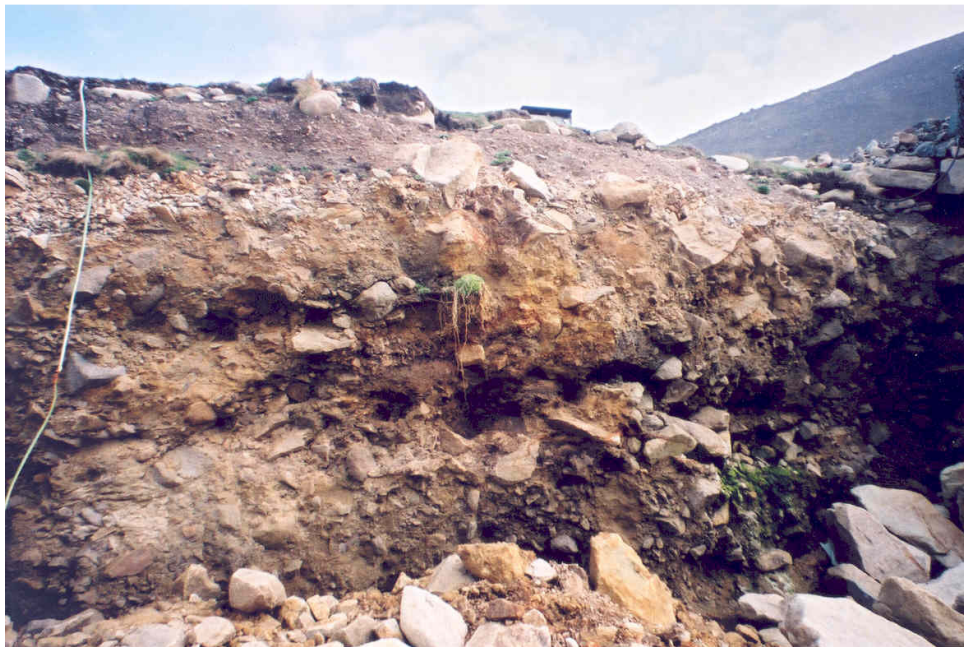
The same section in 2003(STK 03 3/10) The overhang has collapsed and a stone has fallen from the top
