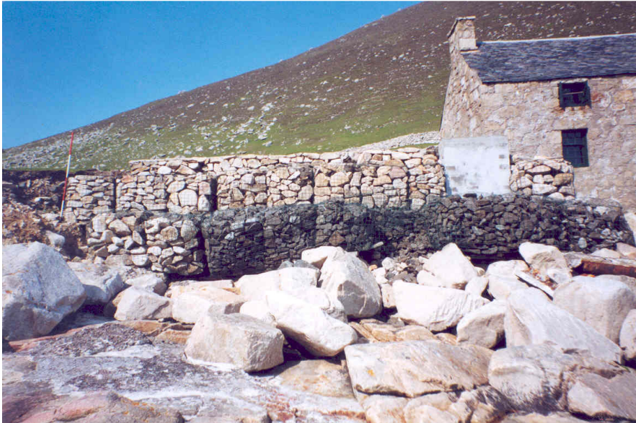
Coastal erosion Section C – 2002 (STK02 9/22)
