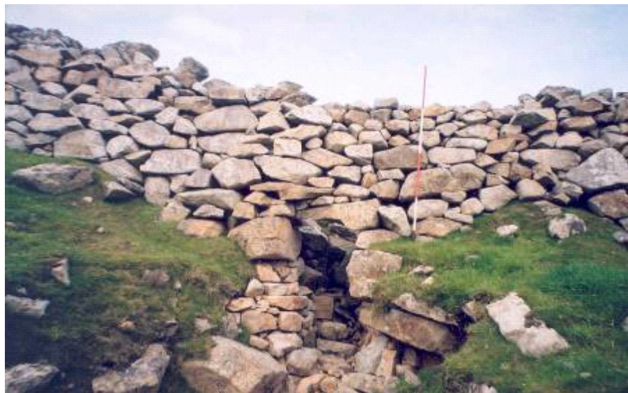
The Dry Burn with the revetment wall on the west side repaired
