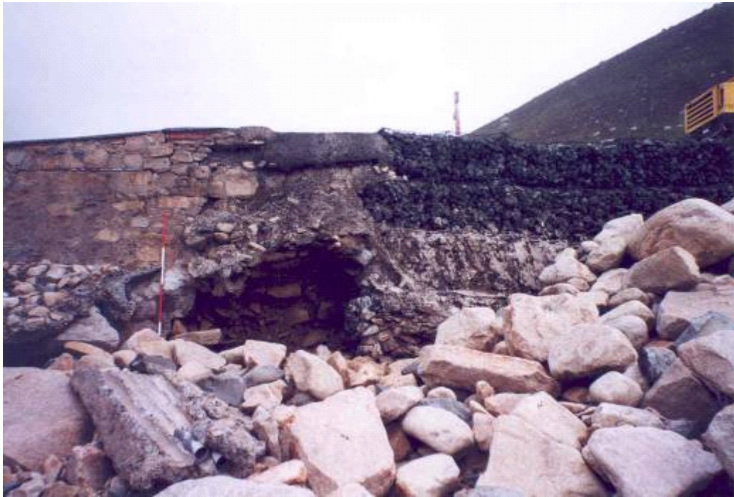
Coastal erosion section C 2002 (STK02 10/23)
