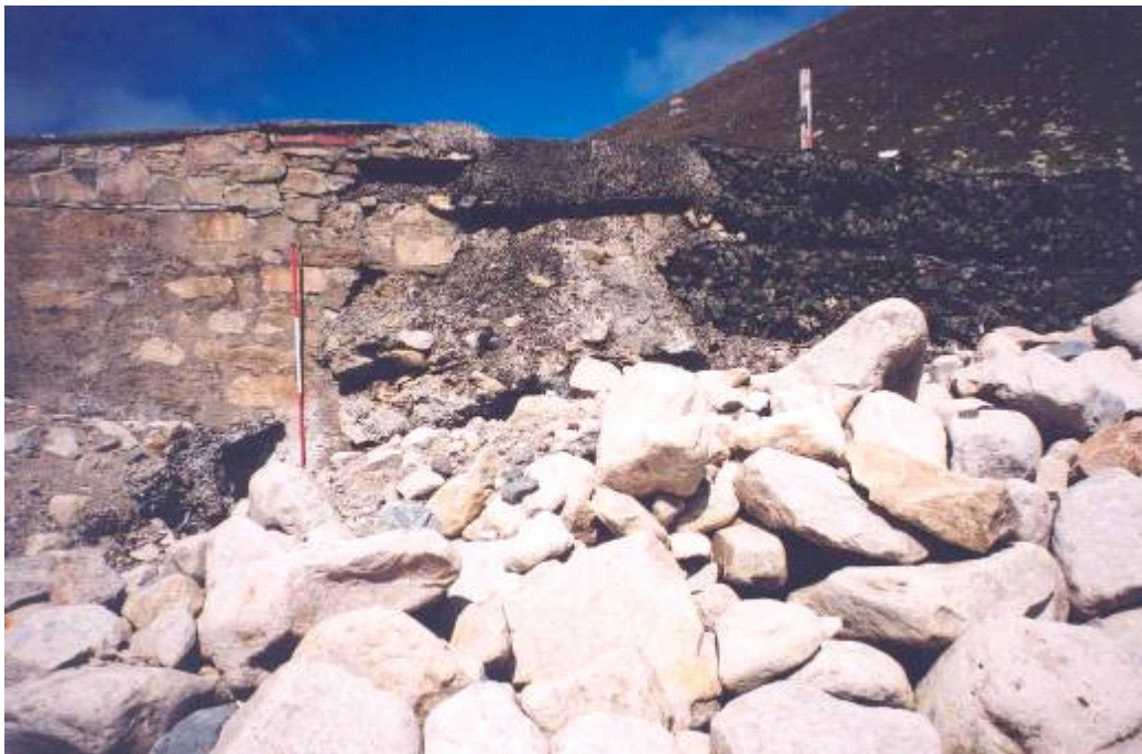
The same section in 2004 (STK04 1/32a). Debris has been deposited in front of the hole under the slipway, hopefully delaying further erosion
