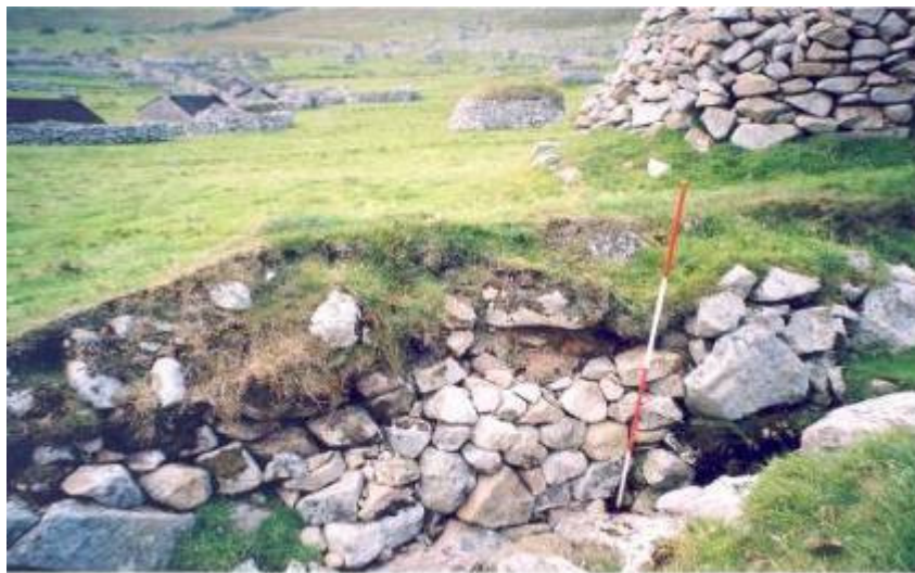
Work continued downstream, rebuilding sides and re-creating a flat base in order to create a sound channel for the water flow and to prevent scouring
