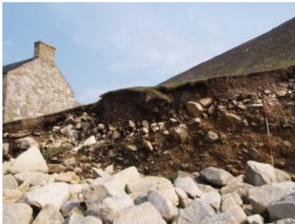
Coastal erosion observed at east end of Village Bay
