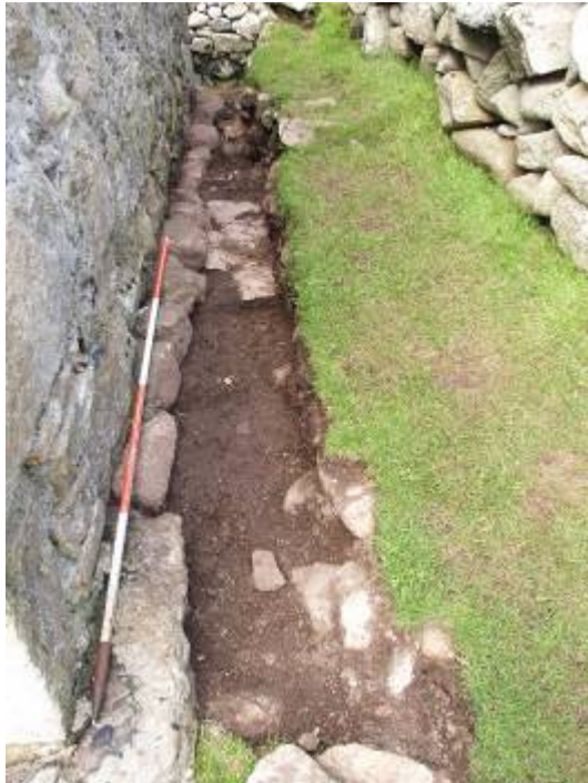
Excavation along the east gable of House 6 in preparation for a new drain
