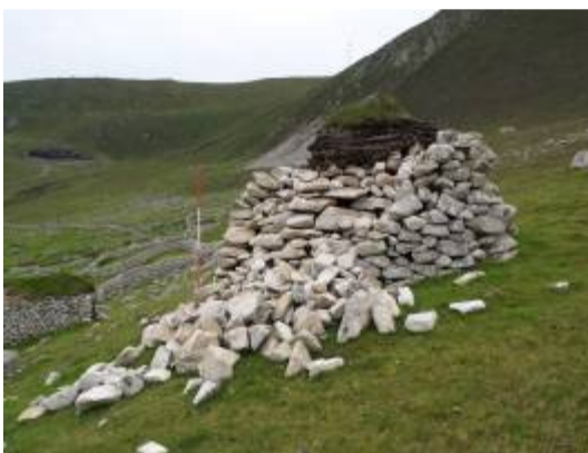
Photo of the major collapse of cleit 168, just beyond the head dyke, taken before its repair in July 2006
