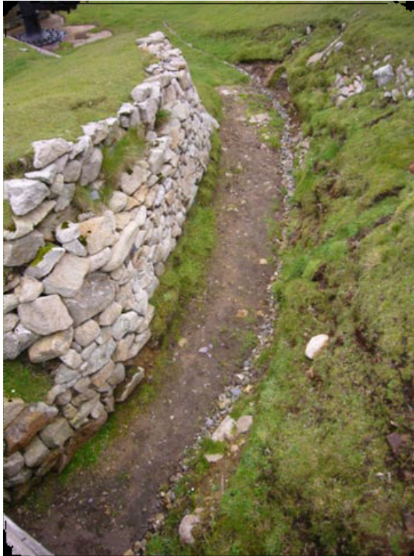
Figure 16 - Munitions Store Drainage
