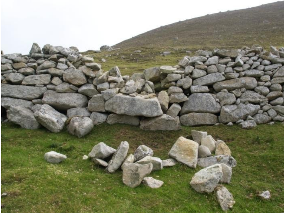
Figure 15. A collapse to the Head Dyke to the north of the Factor's House
