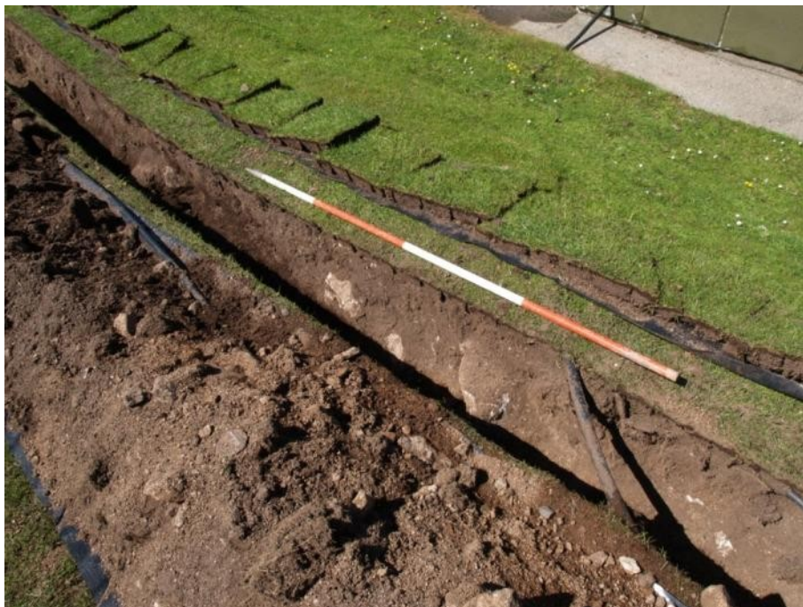
Figure 19. The pipe trench after excavation. No archaeological features, deposits or finds were identified
