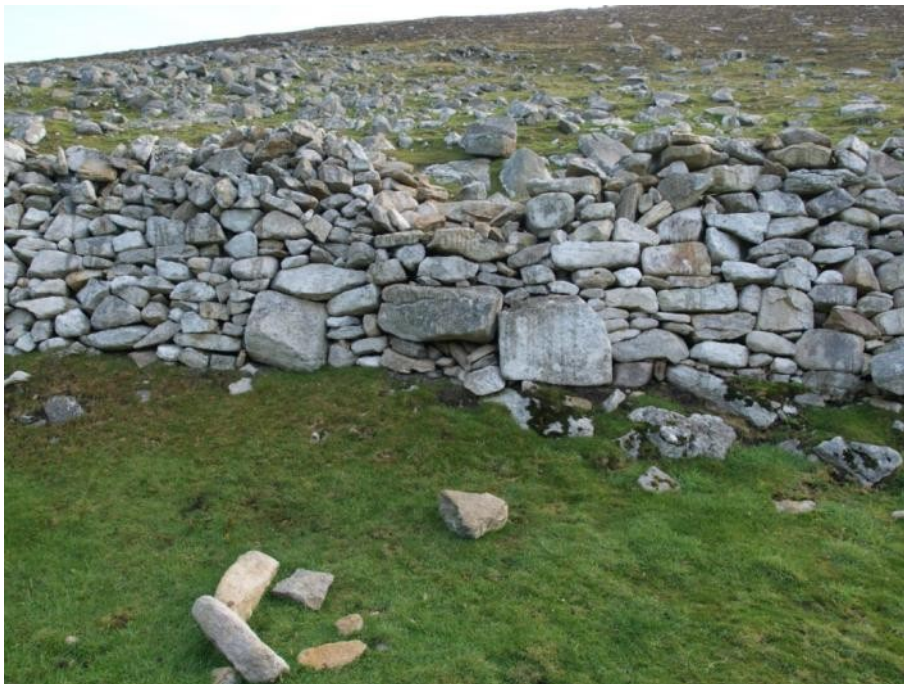
Figure 16. A small collapse to the Head Dyke in Enclosure 2
