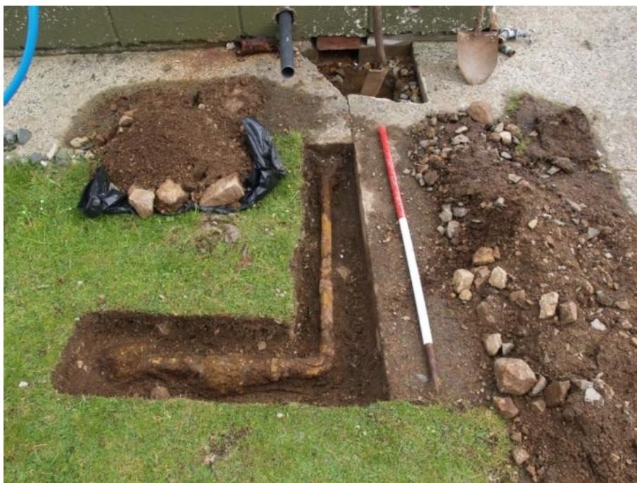
Figure 20. A short section of corroded pipe exposed. The pipe is due to be replaced in 2013 and the excavations will be fully detailed then
