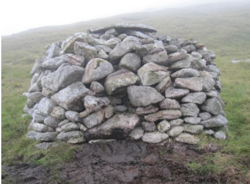
Figure 3. Cleit 686 before (top) and after it collapsed (middle), and after it was repaired by Innes Watson (bottom)
