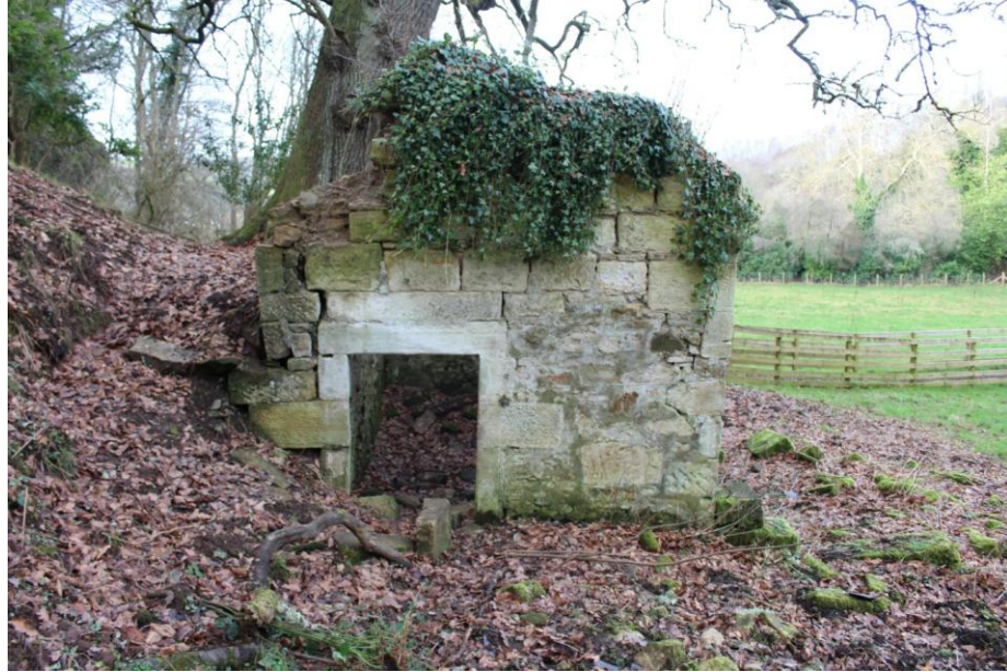
Illus 42: Doorway of the stone built fruit store/tool shed (?) adjacent to Burnetholm Cottage on the furthest edge of Burnetholm Parkland, looking towards the River Clyde. The wooden fencing marks the Clyde Walkway.
