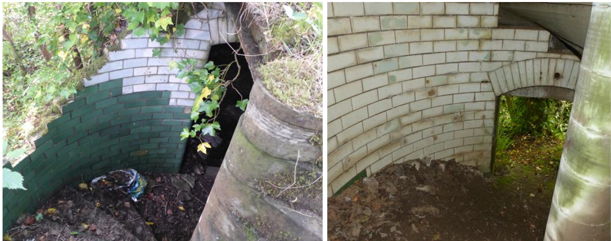
Illus 47: Views of the tiled internal spiral case in what remains of Stonebyres House.
