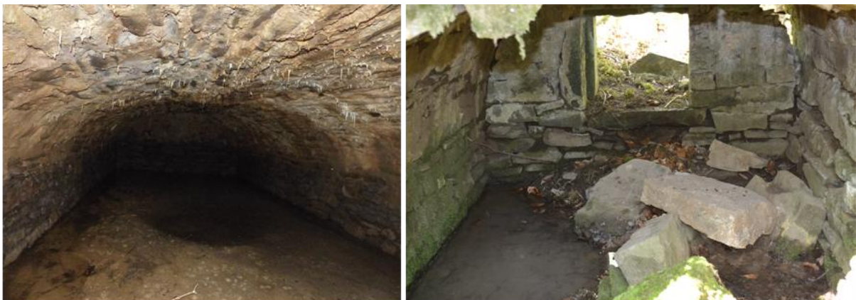
Illus 53: Water tank 1: Left the interior of the upper structure. Right: The interior of the lower structure
