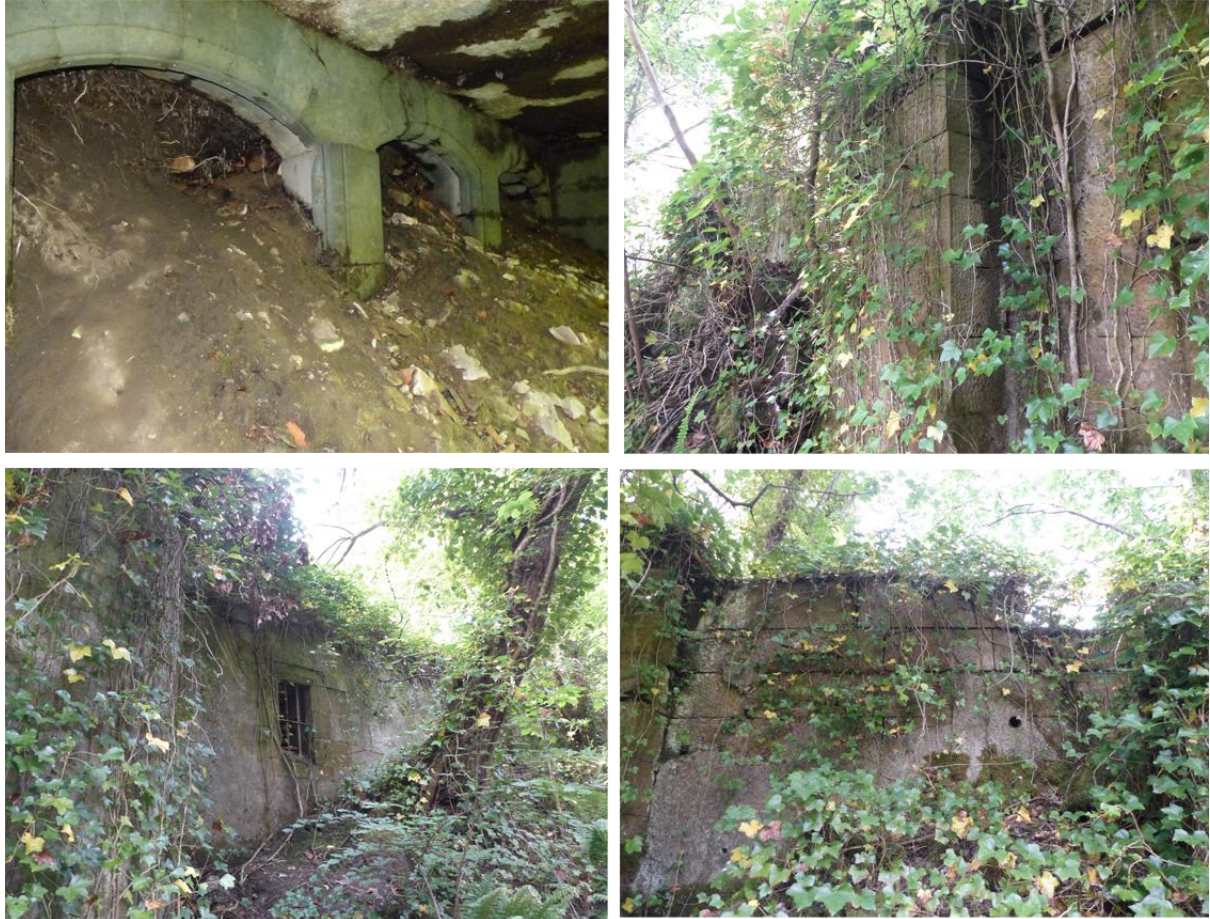
Illus 48: Views of the rooms and wall of Stonebyres House visible below ground level along the burn
