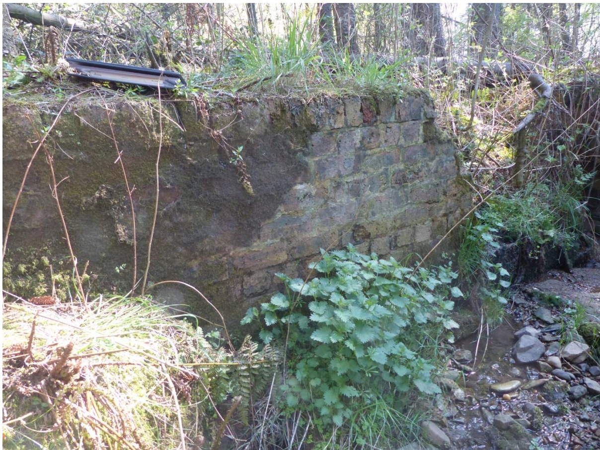
Illus 46: Part of the brickwork in Stonebyres Burn, possibly part the system for controlling the level in the pond. Glorious Gardens: The Development of the Designed Landscape at Stonebyres, Clyde Valley
