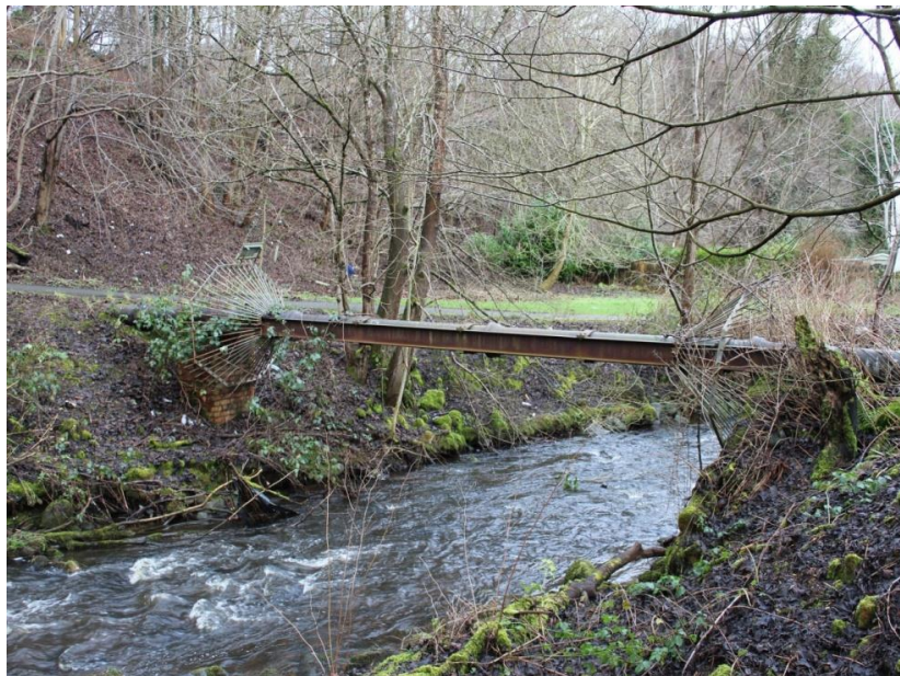
Illus 20: Pipe crossing the burn.
