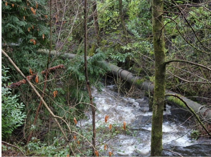
Illus 17: Sewage pipe running alongside burn.
