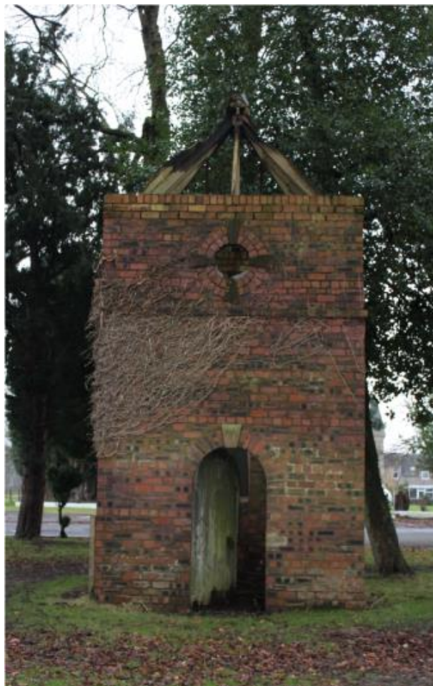
Illus 24: Building to north of house contains pipework and remains of boiler
