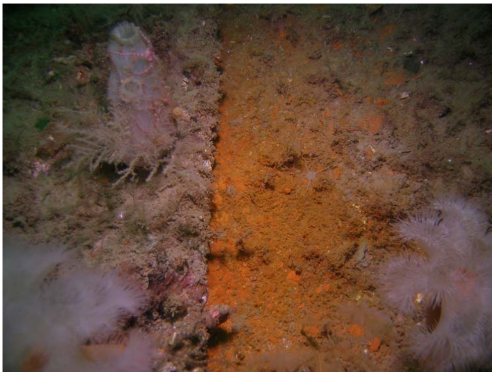
Figure 4.16: Corrosion along overlap indication plates beginning to separate.
