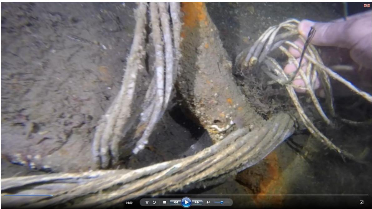
Figure 17: Close up shot of cable showing multiple cores of plastic insulated wires. The corroding steel sheathing on the cable is evident behind.
