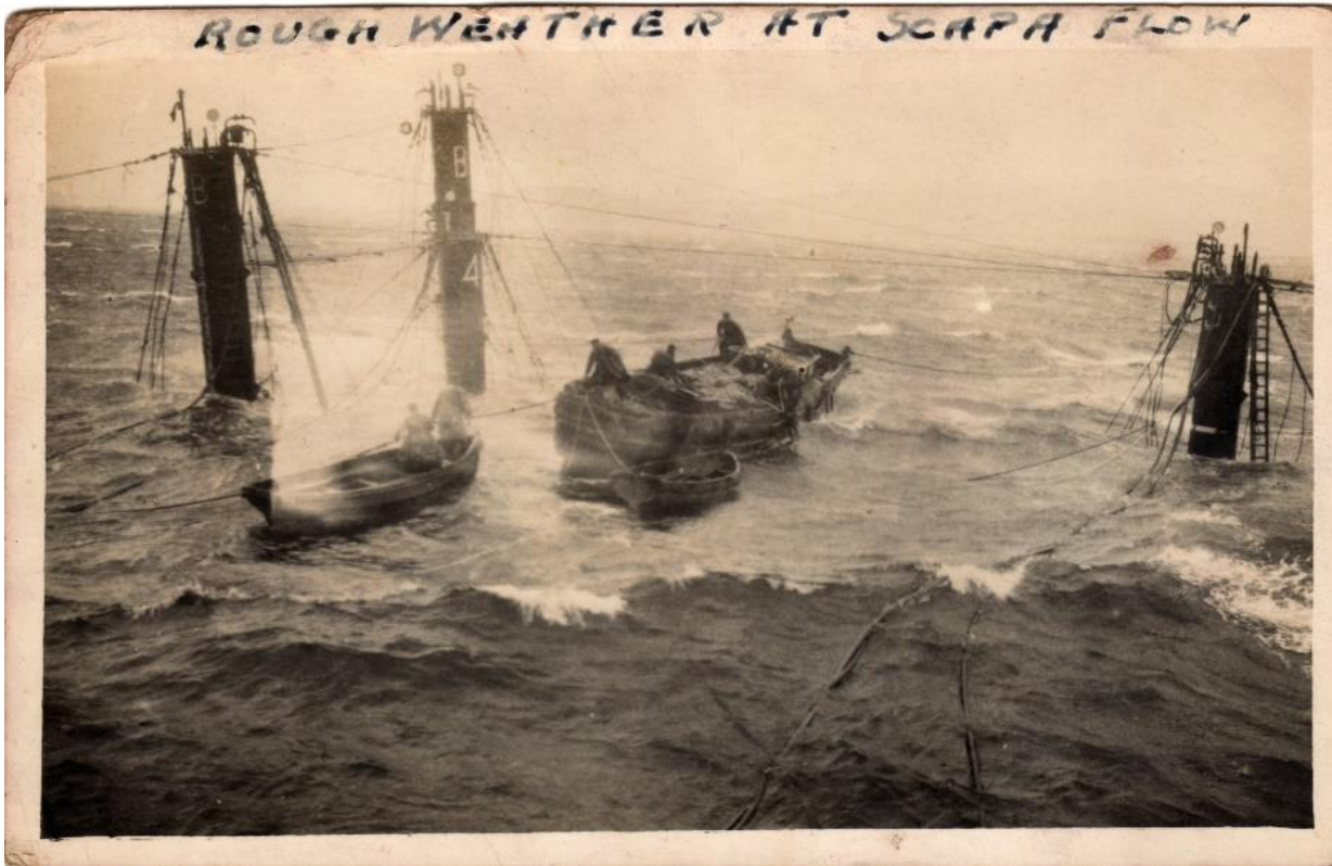
Plate 1: Air locks fitted to the hull of a sunken German vessel (C. Bullen Collection). Workers accessed the air locks by small boats and descended through them to the hulls on the seabed below.
