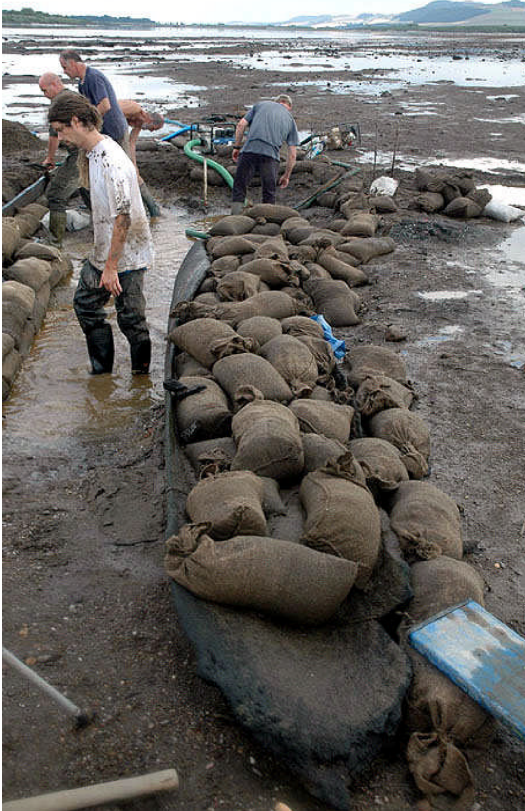
Illus 33: Sandbagging of the interior of the boat for protection during excavation.
