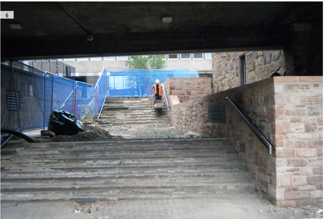
ILLUS 4 SW facing section showing made ground to bottom of excavation ILLUS 5 N facing shot of interior of planter box excavated down to formation level ILLUS 6 SE facing shot of stairs and shelf to be re-surfaced. New wall built during Phase 1 to the right. Phase 2 area between heras fence and outer wall to the left
