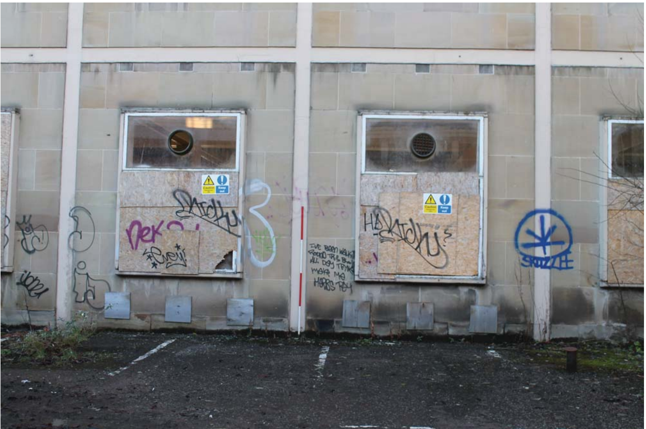
Plate 14: East Wing, detail of the ground floor windows of the north elevation, from the north
