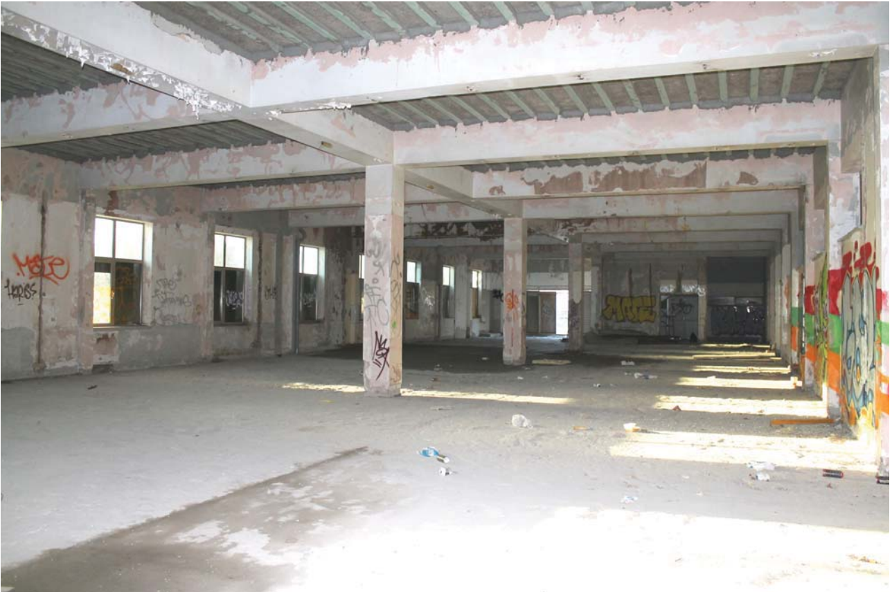
Plate 19: West Wing, ground floor, general view of the interior from the north-east
