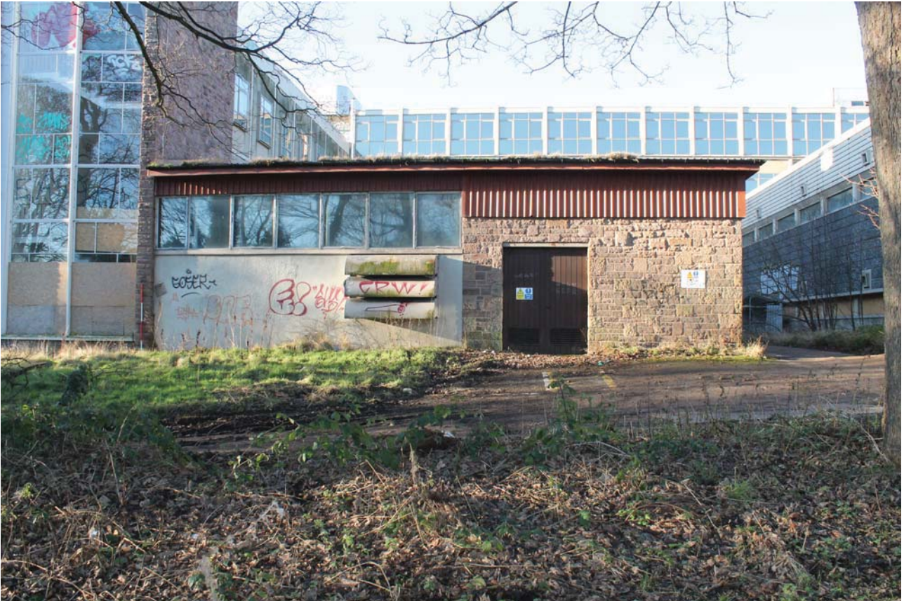
Plate 11: East Wing, general view of east elevation of the single-story block to the north side, from the east
