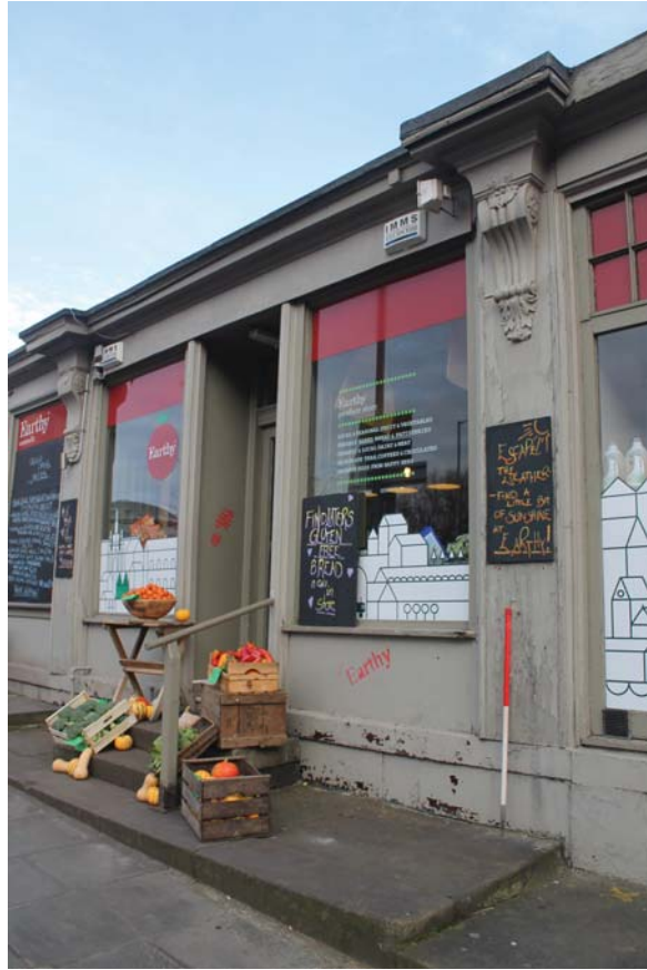
Plate 3: Nos 1 – 6 Canonmills Bridge, detail of the main shop front (second from the south-east) from the south
