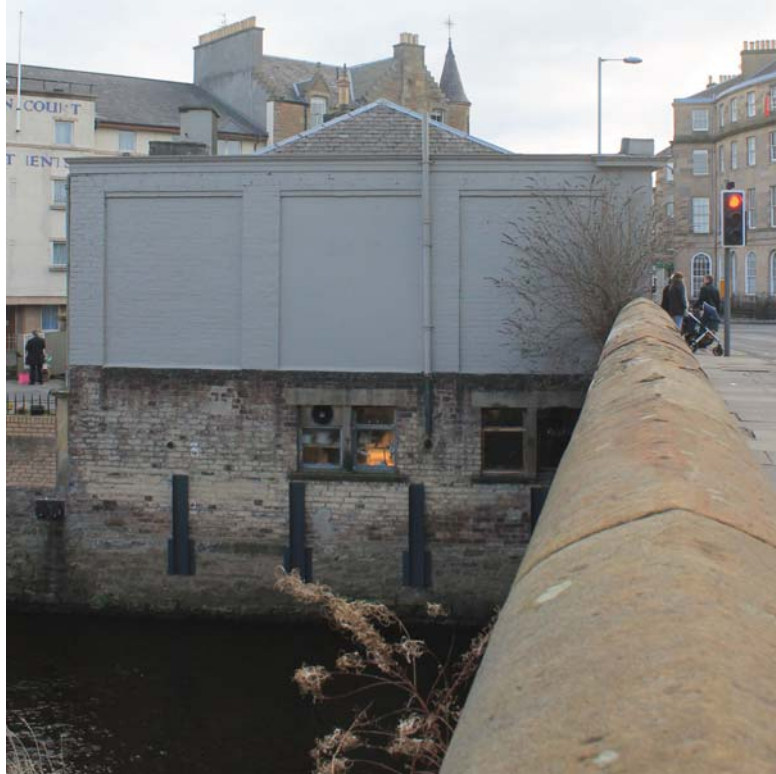
Plate 5: No 1 Canonmills Bridge, general view of the north-west elevation to the Water of Leith, from the north-west
