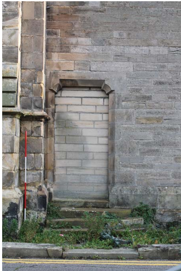
Plate 32: South-west elevation, detail of bricked-up doorway on the south-east end from the south-west
