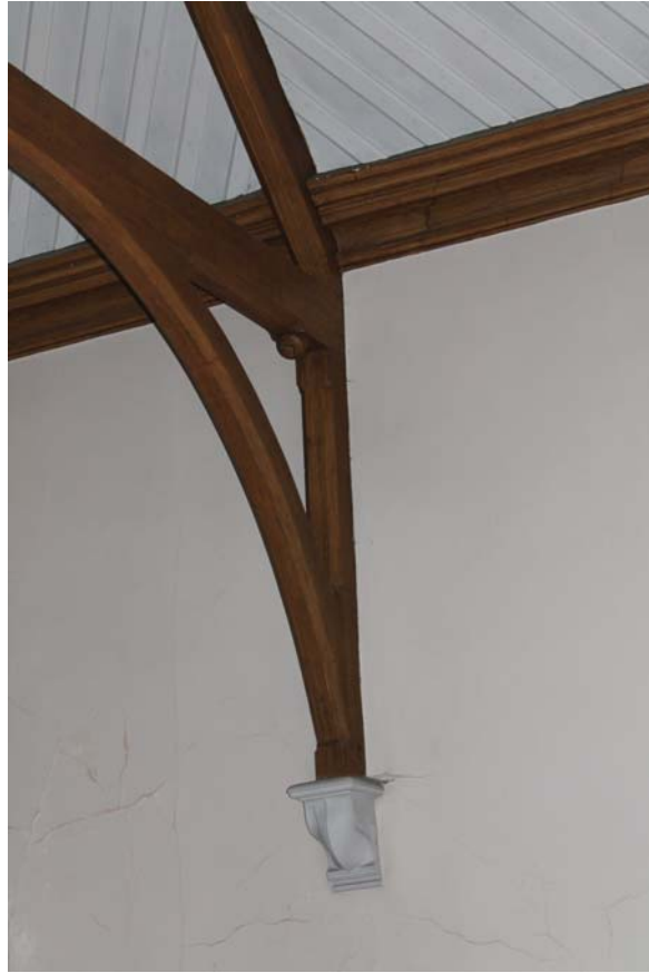
Plate 69: Room 1/1, detail of corbel and base of rafter on the south-west wall from the north
