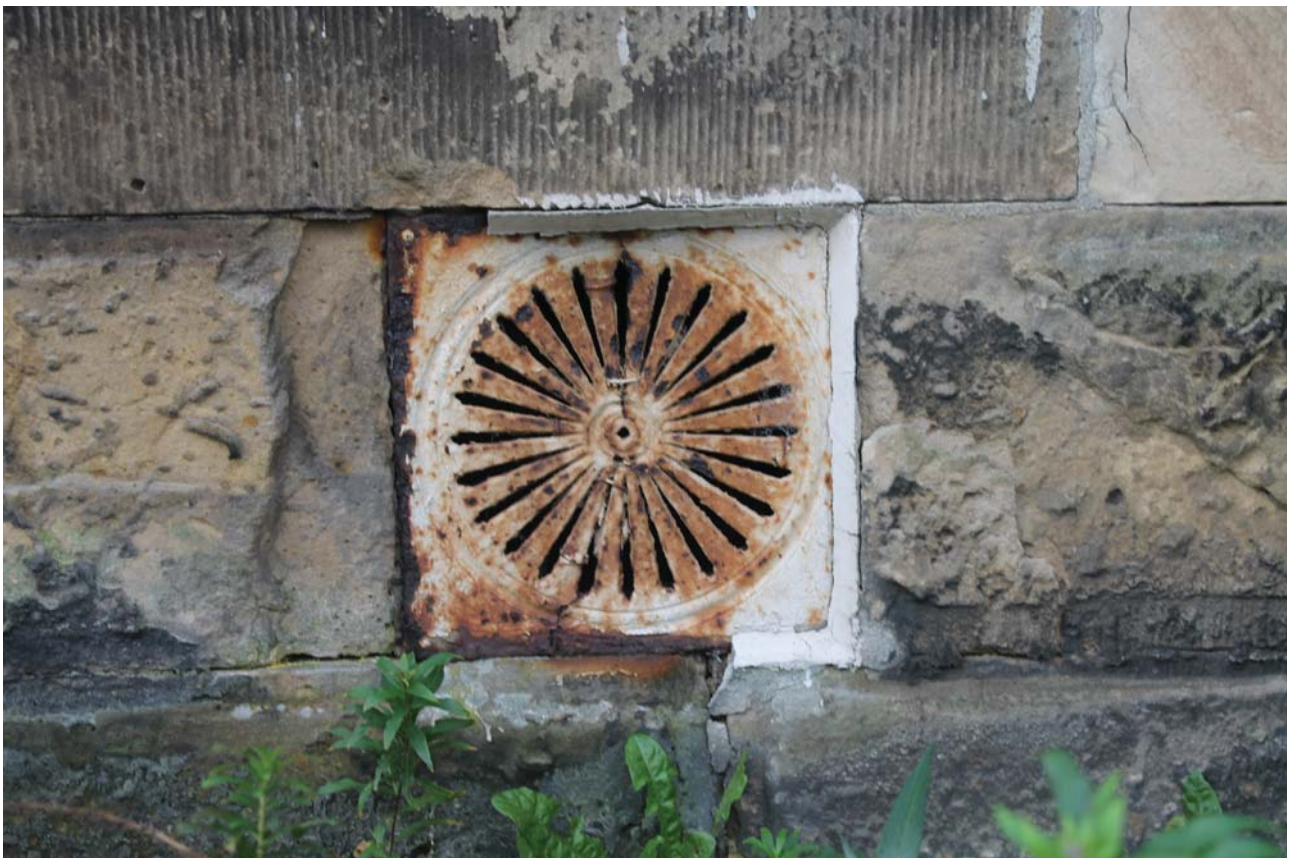
Plate 34: South-east elevation, detail of vent on the original building from the south-west
