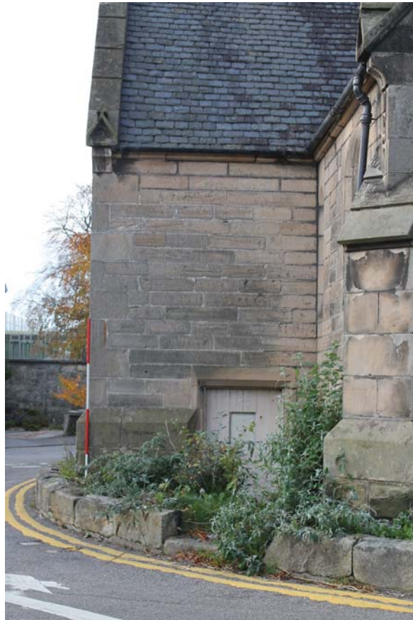
Plate 37: North-east elevation, general view of the later 19th century extension and doorway to the basement from the north-east
