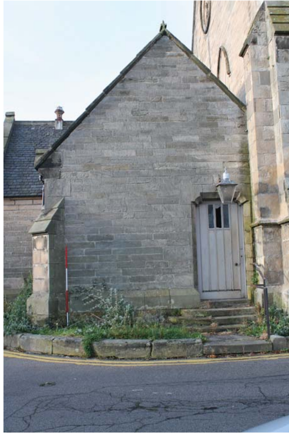
Plate 31: North-east elevation, general view of the south-east end showing doorway through to the small corridor 0/2, from the north-east
