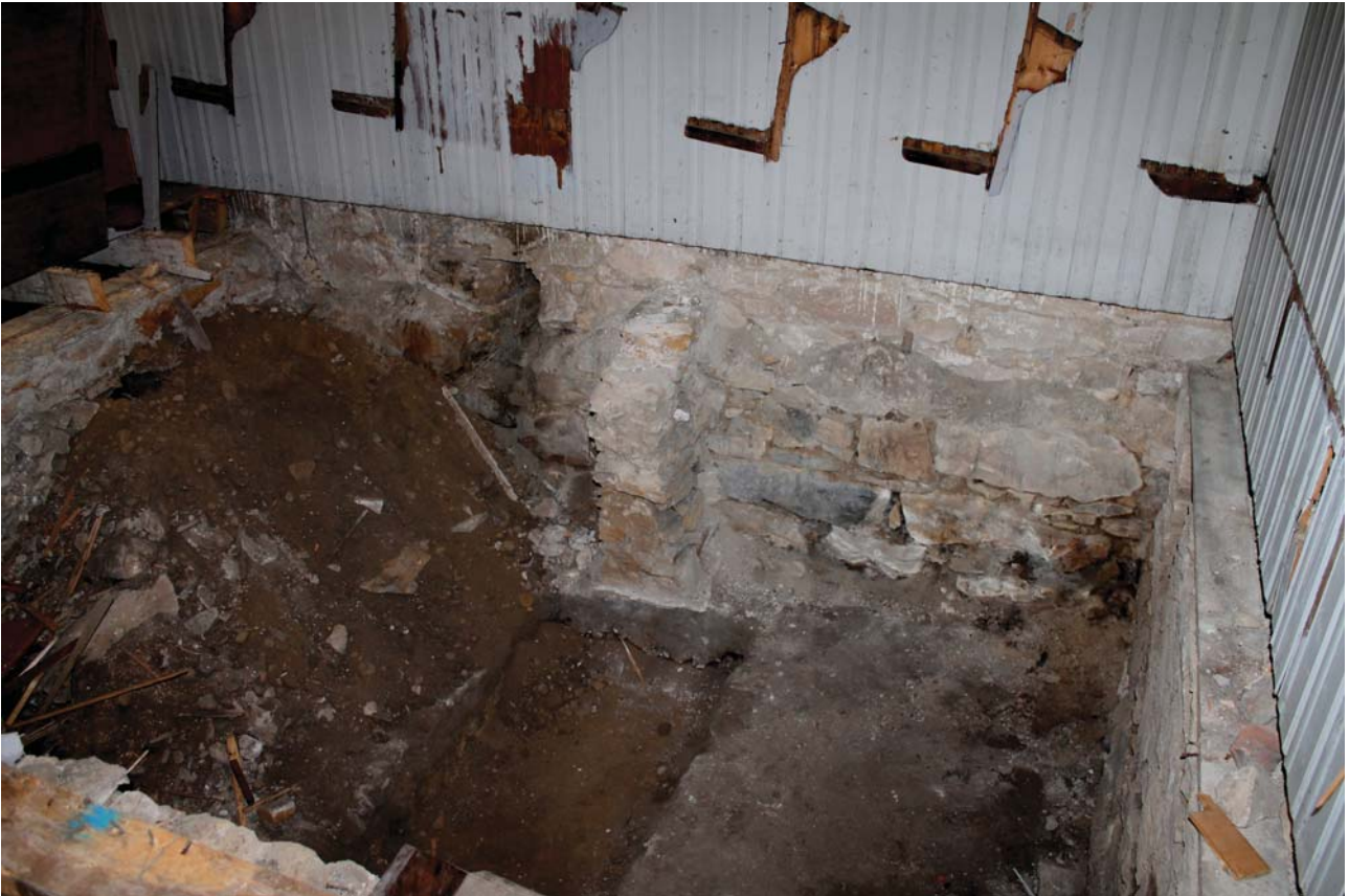
Plate 45: Room 0/1, detail of the excavation trial pit in the western corner showing the stone foundation walls from the NNE
