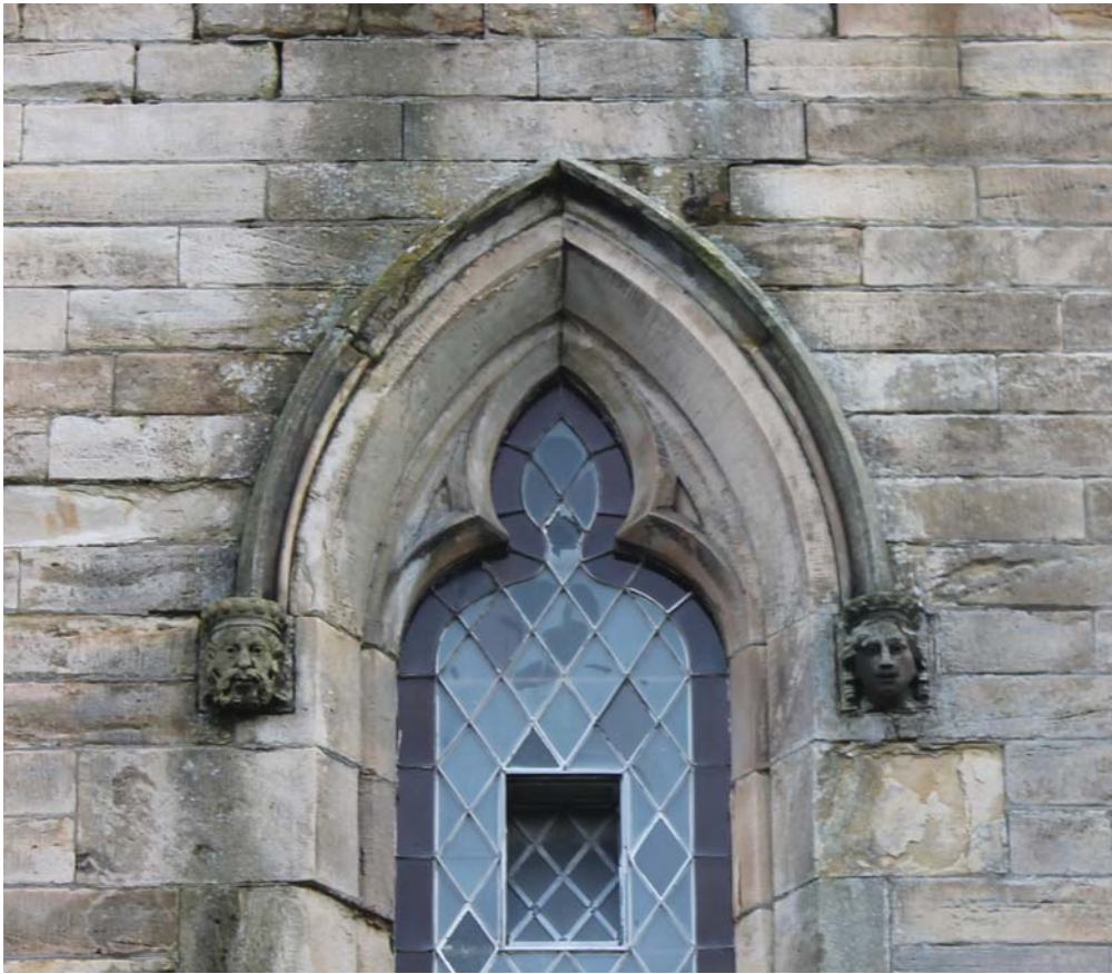
Plate 25: South-west elevation, detail of hood mould over central window from the south-west
