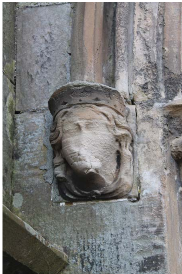
Plate 10: South-east elevation, detail of the carved figure/stop to the hood mould on the main doorcase on the north-east side, from the north-west
