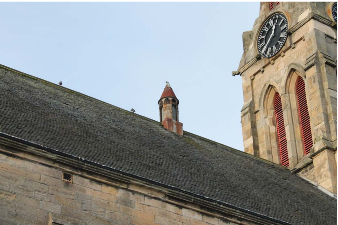
Plate 36: Detail of vent on the apex of the roof of the main body of the church for the east
