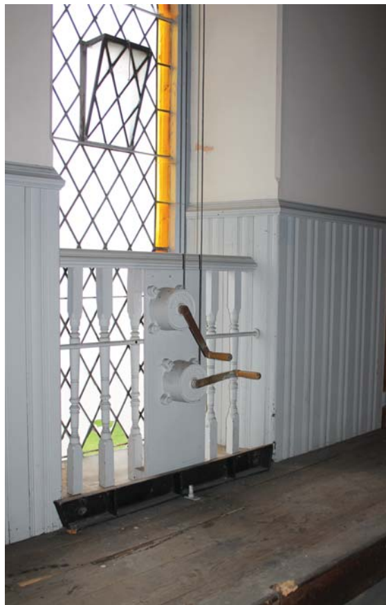
Plate 72: Room 1/1, detail of mechanism for operation of the ventilation system in front of window in the north-east wall from the west
