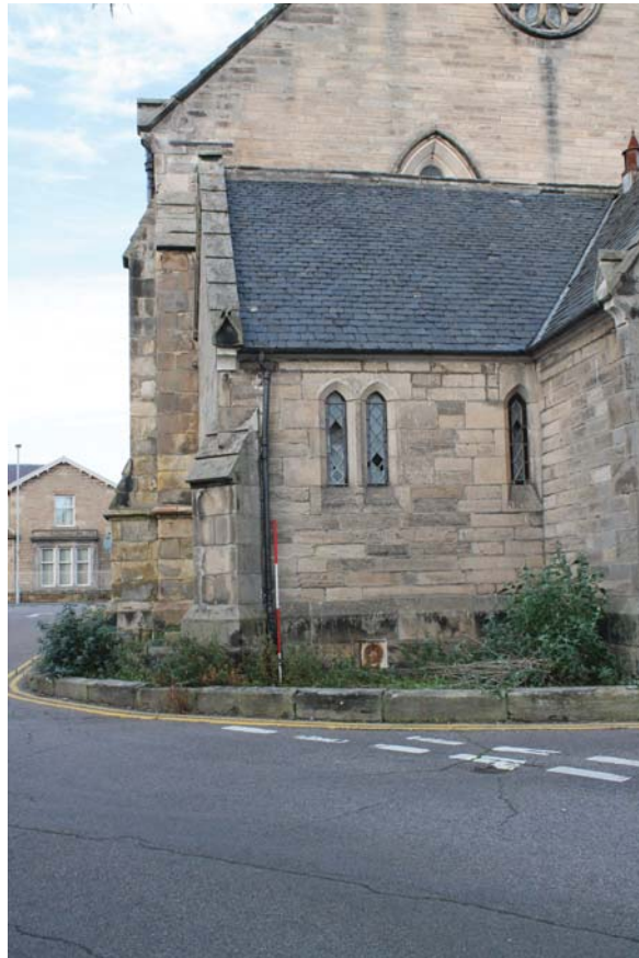
Plate 33: South-east elevation, detail of the windows to the south-west side from the south-east
