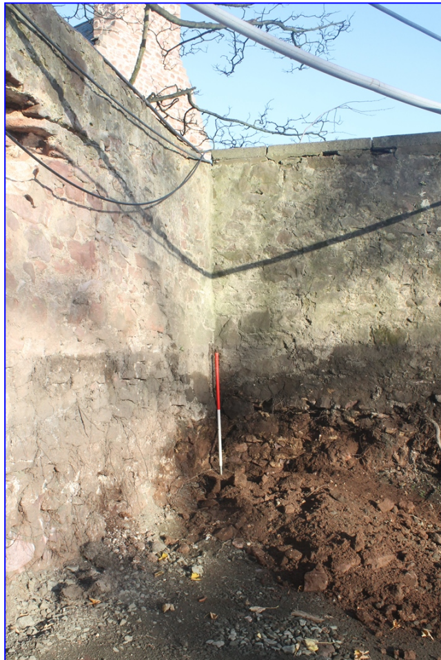
Plate 4: Detail of junction between original wall (left) and later building (east) from the south
