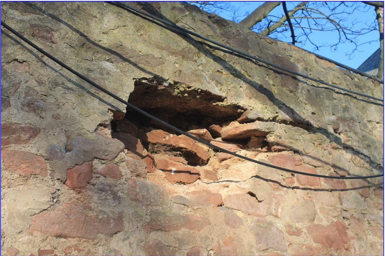
Plate 5: Detail of broken away area of stonework to the top of the west wall from the south-west
