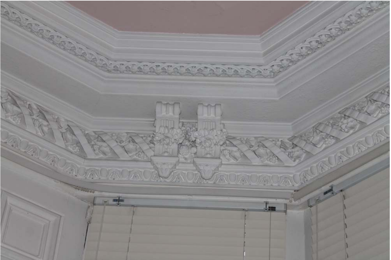
Plate 77: Room 0/7, detail of cornice showing console brackets on the south wall from the north
