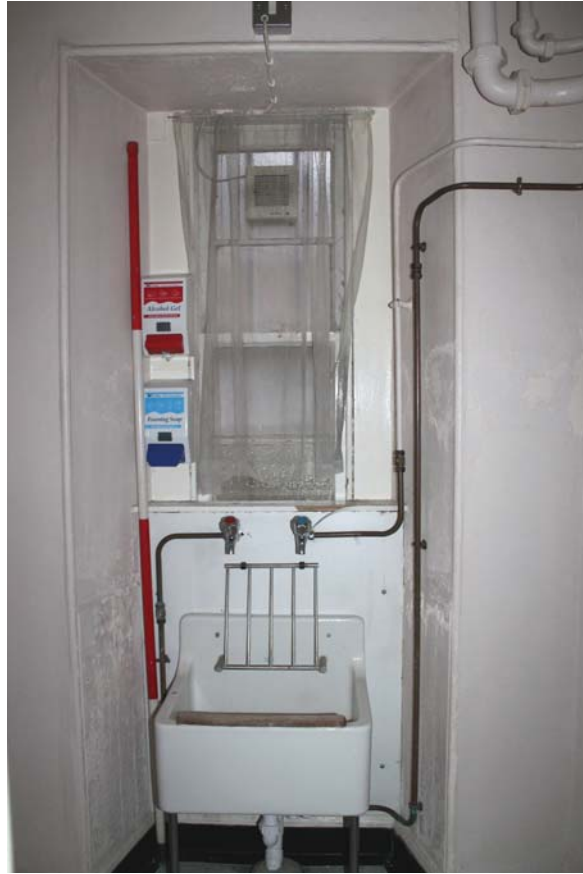
Plate 51: Room 0/2, detail of the window in the westernmost 'cupboard' (now forming a small washroom), from the south-east
