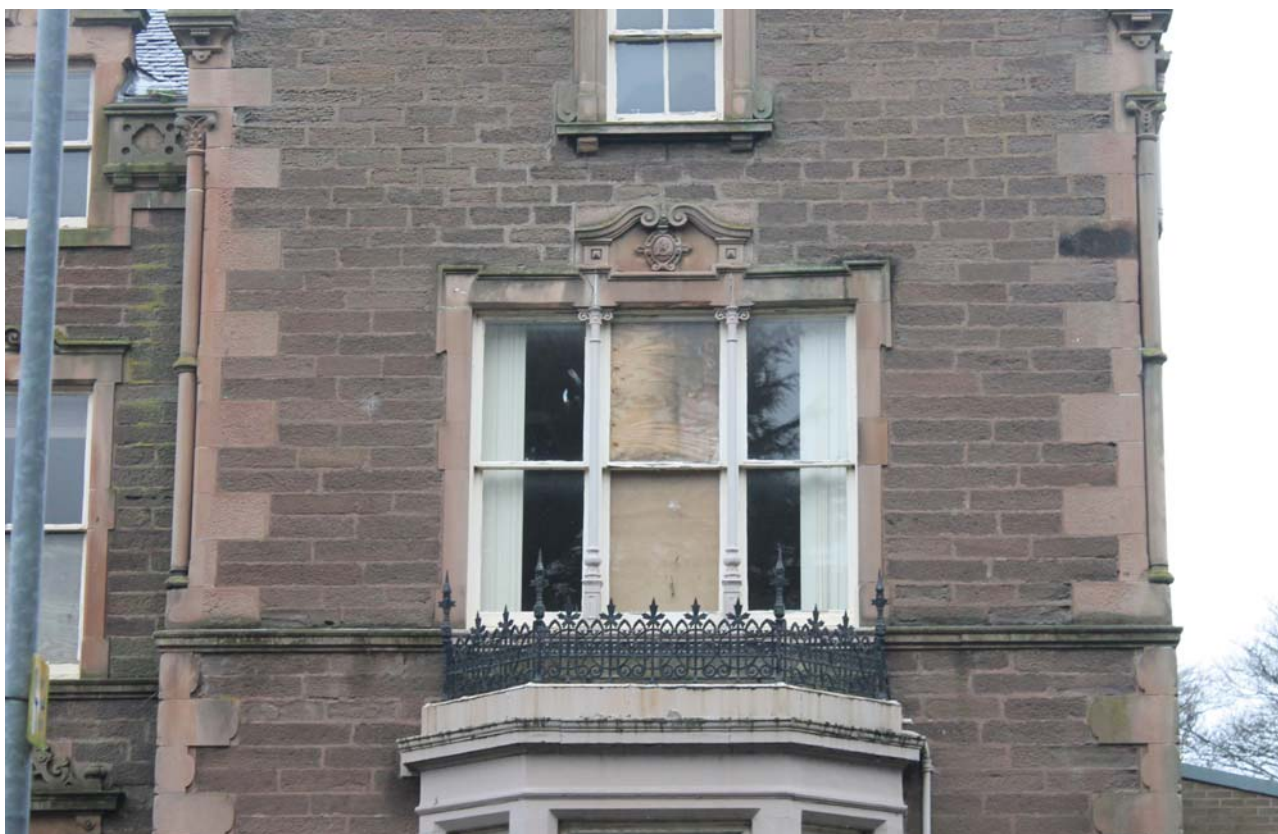
Plate 17: Ashludie House, South Elevation, detail of the first floor of the eastern gable from the south
