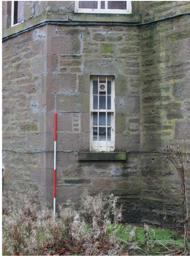
Plate 25: Ashludie House, North Elevation, detail of ground floor window to the centre bay from the north-west
