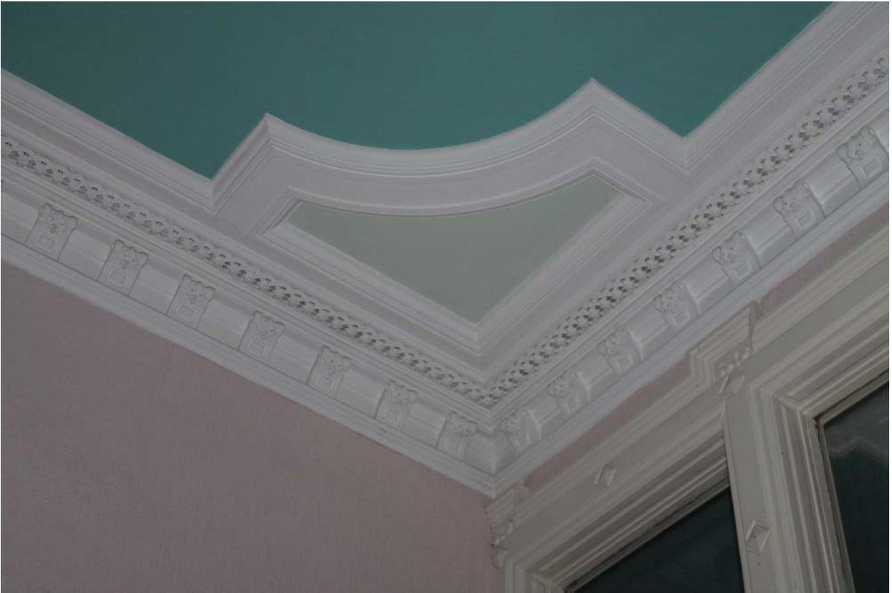
Plate 41: Room 0/1, detail of the decorative ceiling in the north-west corner from the south-east
