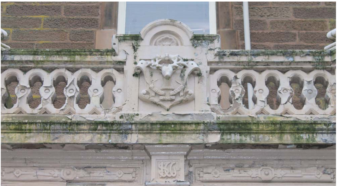
Plate 6: Ashludie House, South Elevation, detail of balustrade above the portico from the south
