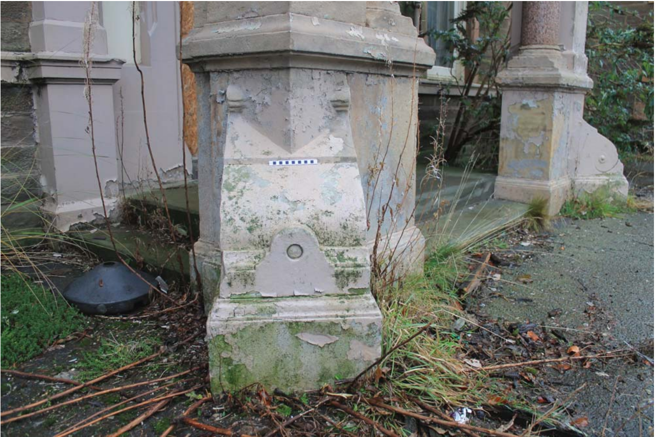
Plate 11: Ashludie House, South Elevation, detail of the footings on the west side from the south-west
