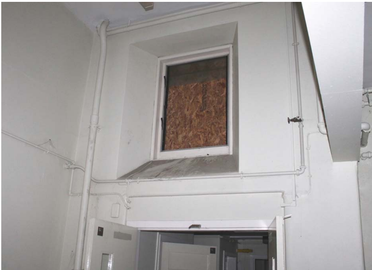
Plate 82: Room 0/10a, detail of upper level window to the north wall from the SSE
