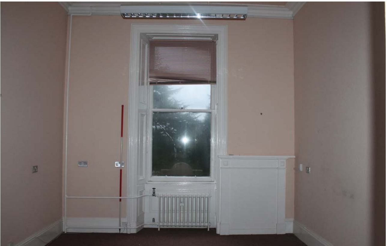
Plate 86: Room 1/3, general view showing window and fireplace in the south wall from the north
