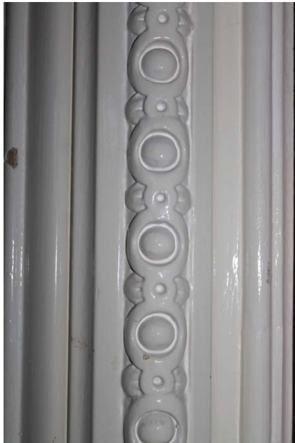
Plate 80: Room 0/8, detail on the side of the door in the east wall from the west
