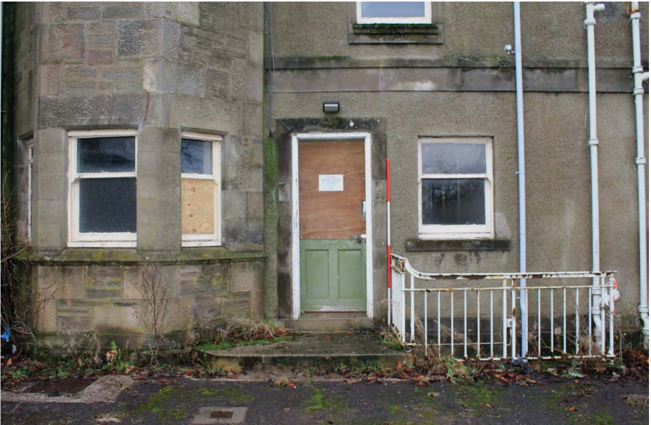
Plate 129: Building B2, East Elevation, general view of the ground floor from the east
