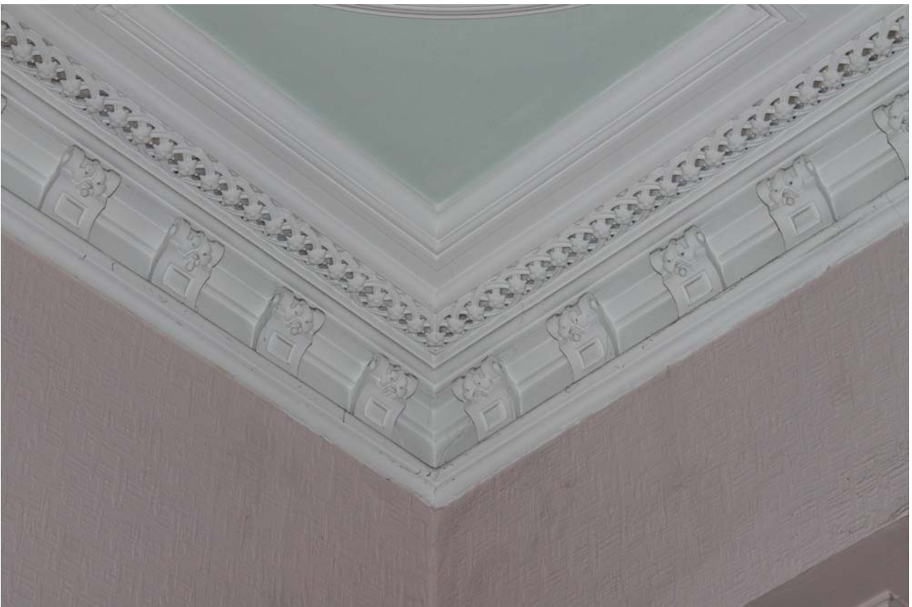
Plate 42: Room 0/1, detail of cornice from the in the north-west corner from the south-east
