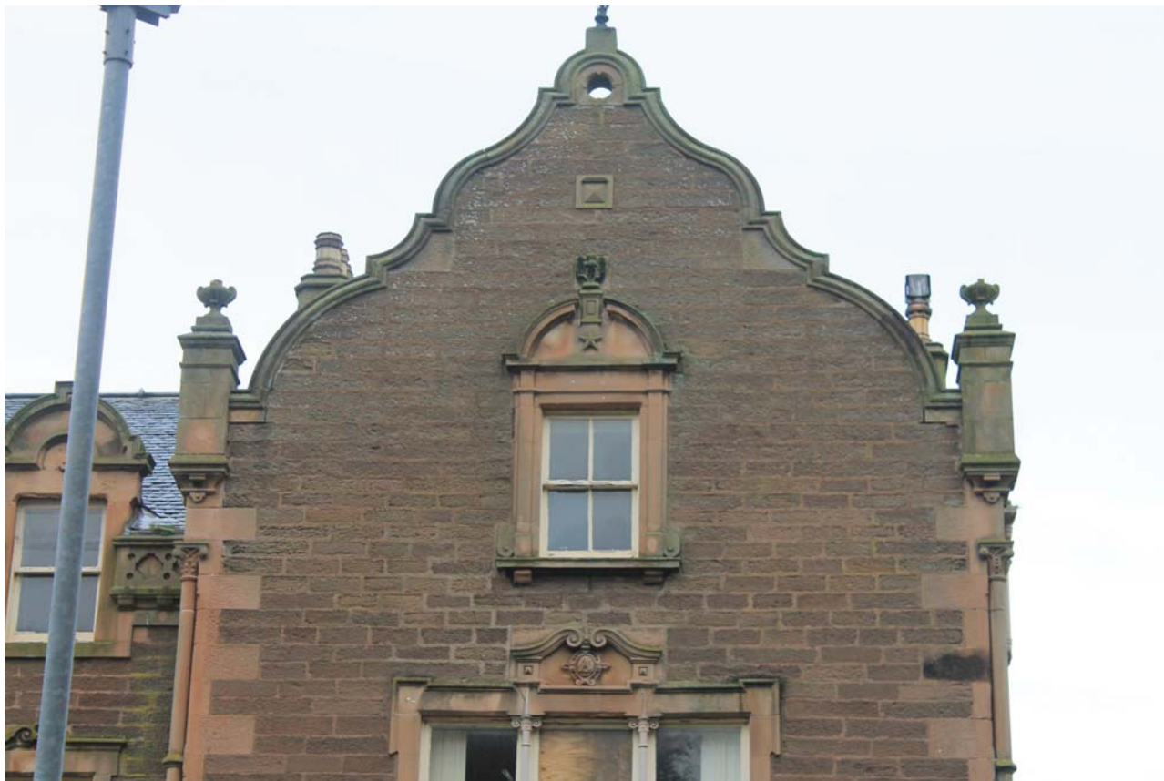
Plate 18: Ashludie House, South Elevation, detail of second floor window on the eastern gable from the south
