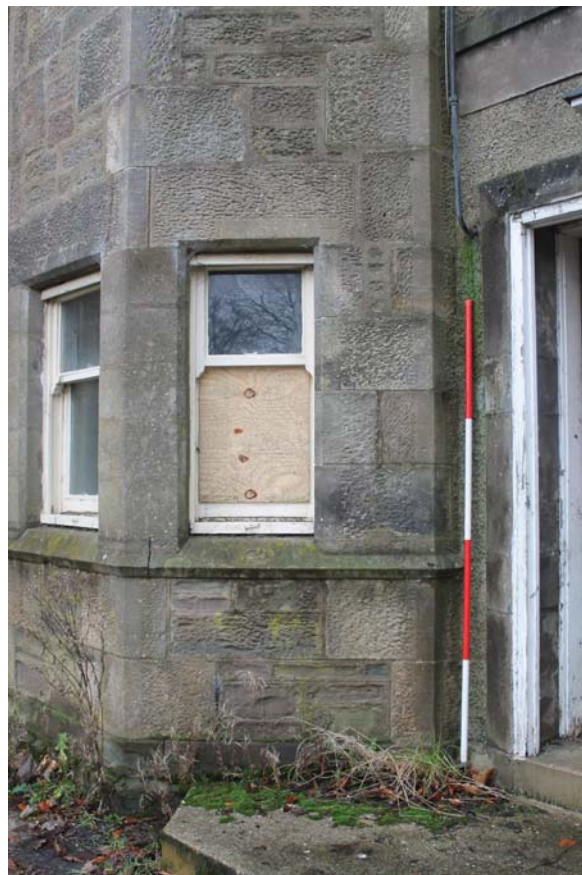
Plate 130: Building B2, East Elevation, detail of window in the north-east angle of bay window from the north-east
