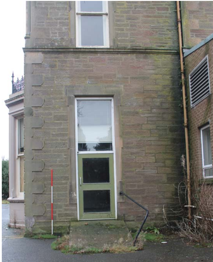
Plate 33: Ashludie House, East Elevation, detail of southernmost ground floor bay from the east
