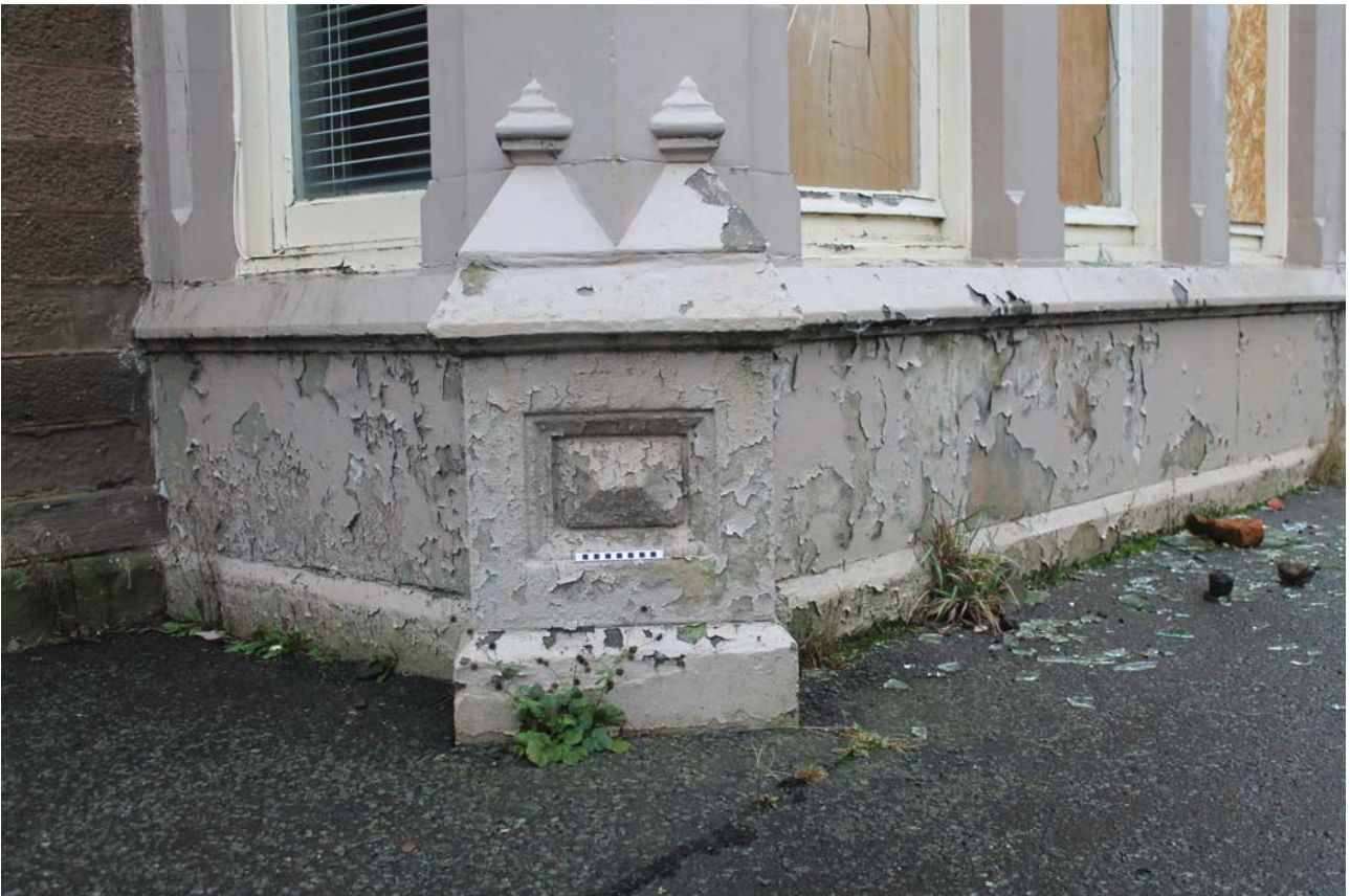
Plate 22: Ashludie House, South Elevation, detail of footing of the bay window to the western gable from the south-west
