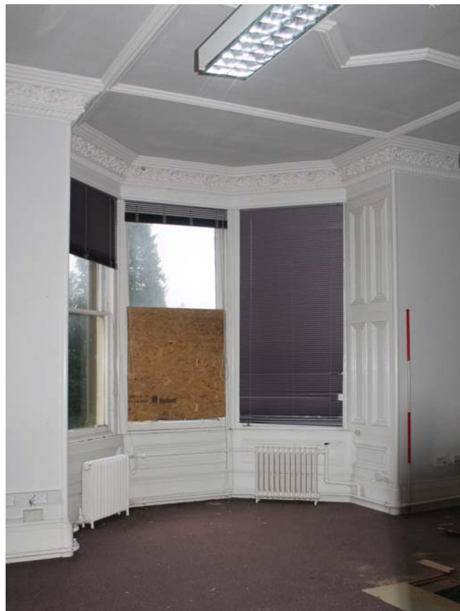
Plate 88: Room 1/16a, general view showing bay window in the south wall from the NNE
