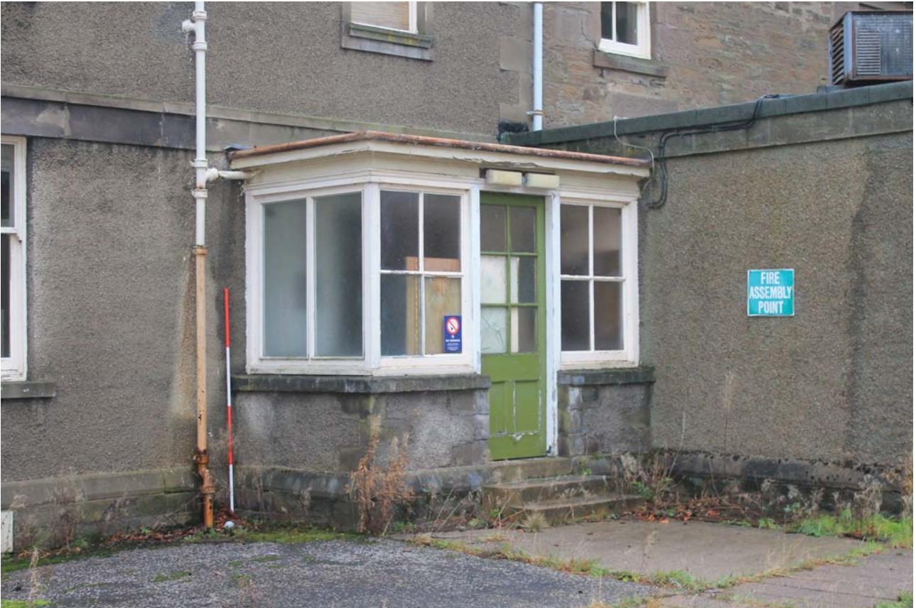
Plate 161: Building D, North Wing, West Elevation, detail of porch to the south side from the north-west
