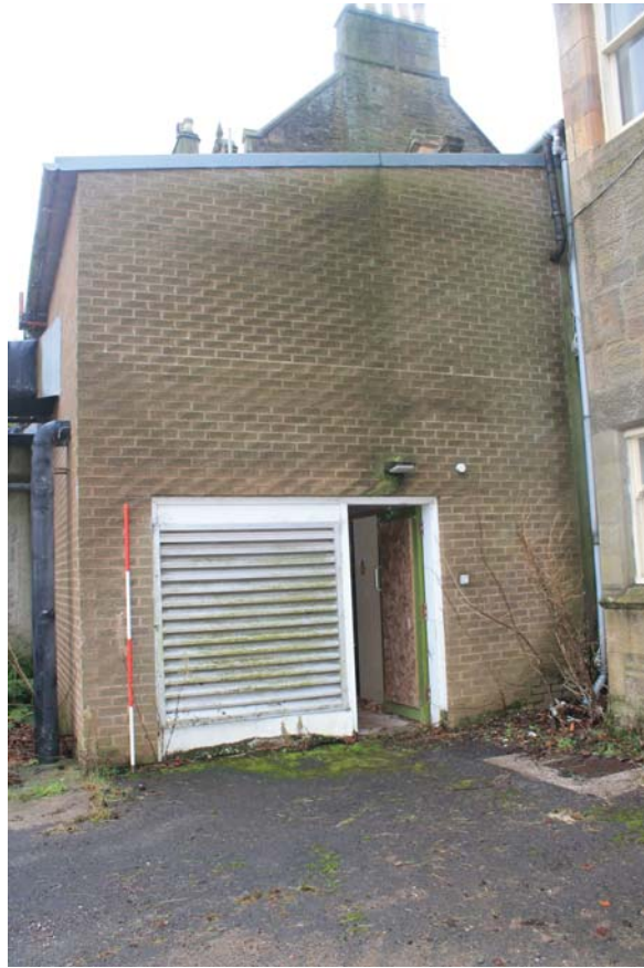
Plate 147: Building C, East Wing, North Elevation, detail of the westernmost bay showing the later modern lean-to, from the north
