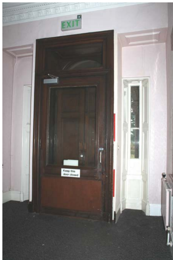
Plate 36: Room 0/1, detail of main door to the south wall from the NNE
