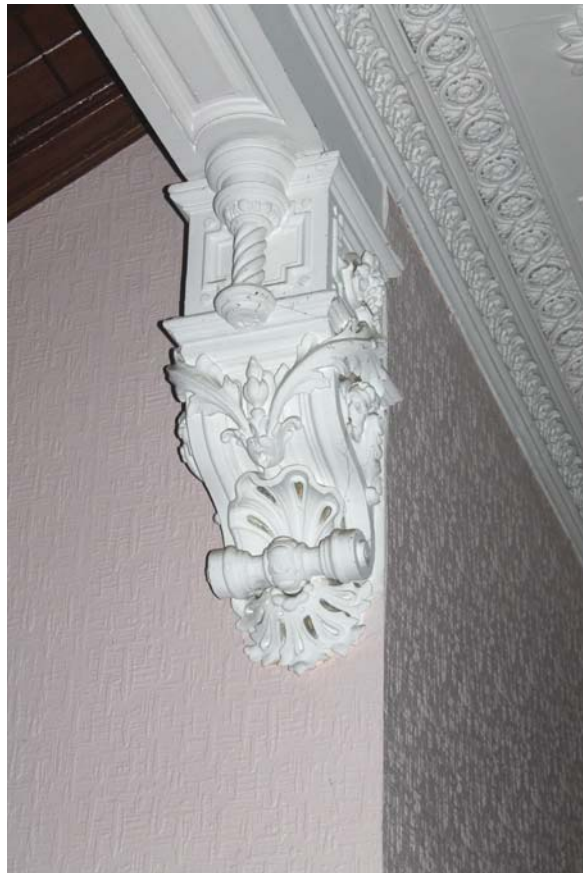
Plate 52: Room 0/2, detail of console bracket to the east side of the stair from the south-west
