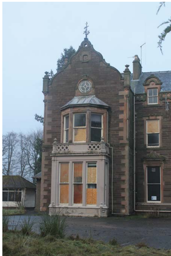
Plate 20: Ashludie House, South Elevation, general view of the western gable from the SSW
