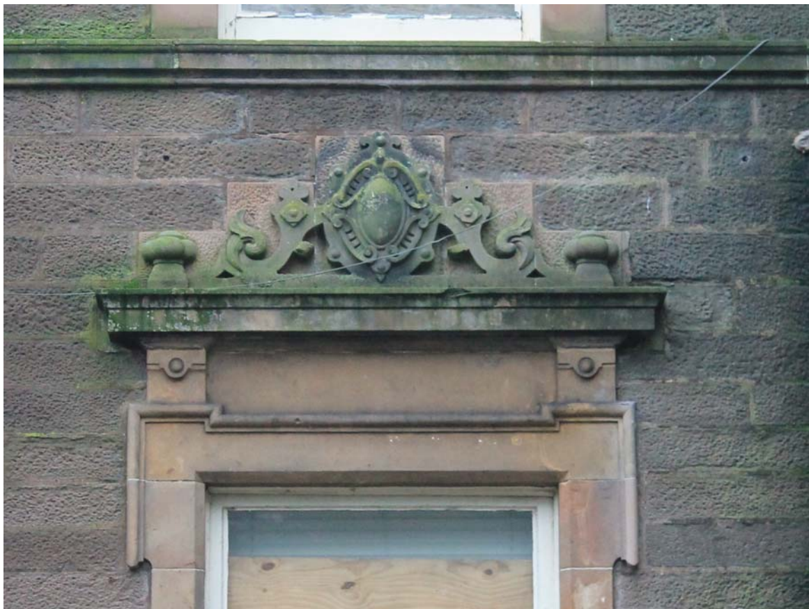
Plate 4: Ashludie House, South Elevation, detail of top of window to the centre bays from the south
