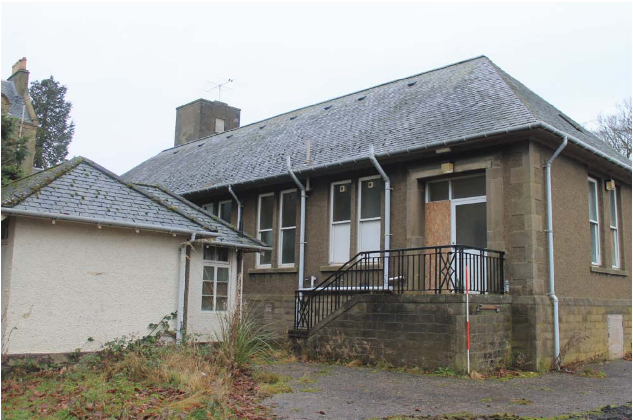
Plate 144: Building C, East Wing, South Elevation, detail of easternmost bay from the south-east
