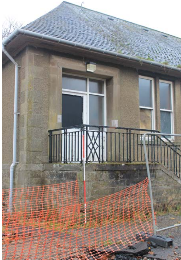
Plate 143: Building C, East Wing, North Elevation, detail of easternmost bay from the north-east
