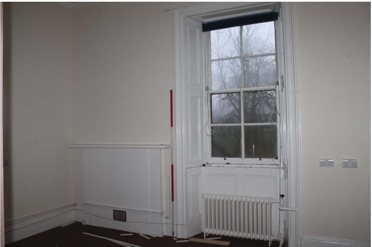
Plate 100: Room 1/9, general view showing window and fireplace in the north wall from the south-east
