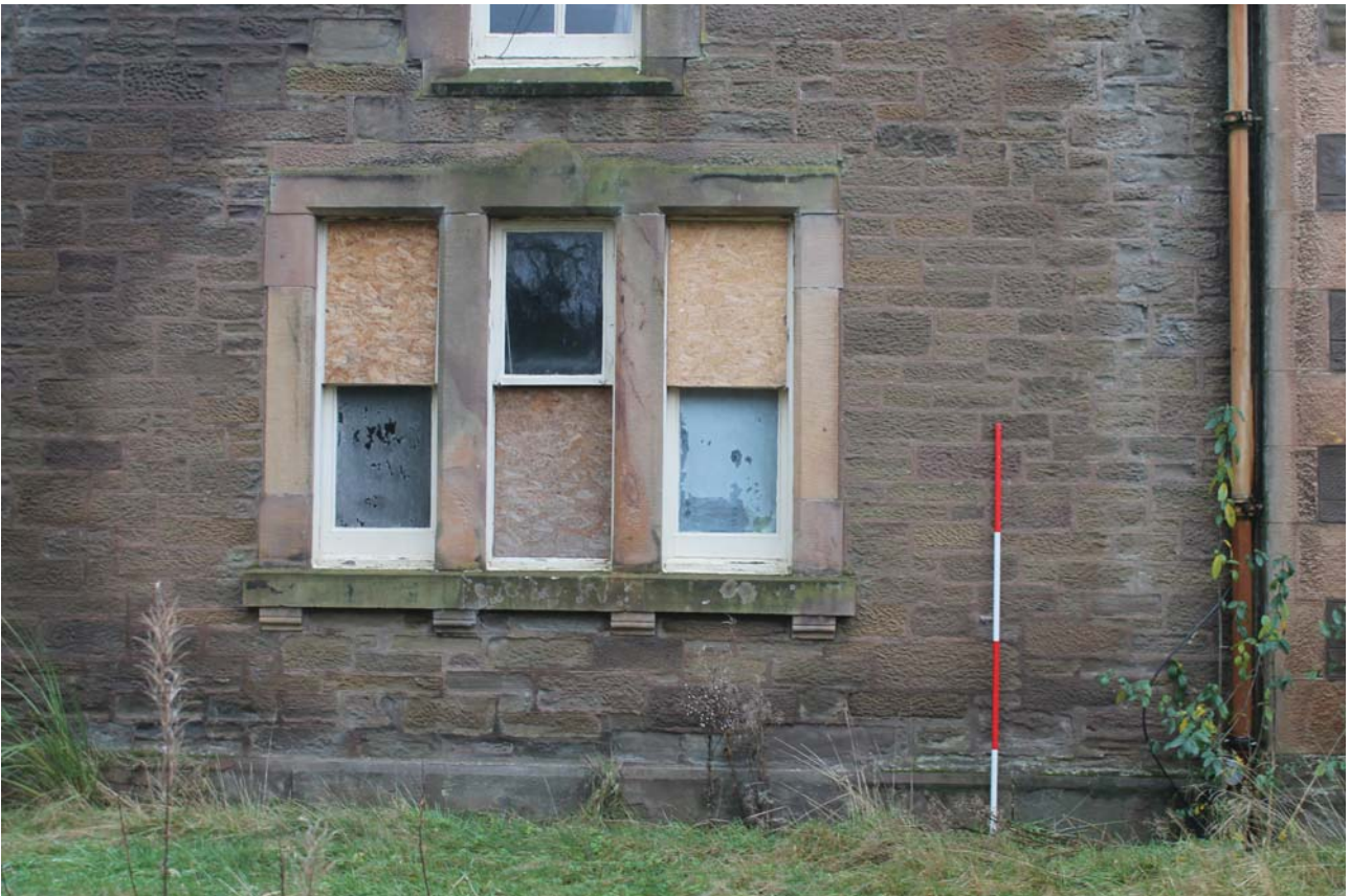
Plate 124: Building B1, West Elevation, detail of ground floor tripartite window from the west
