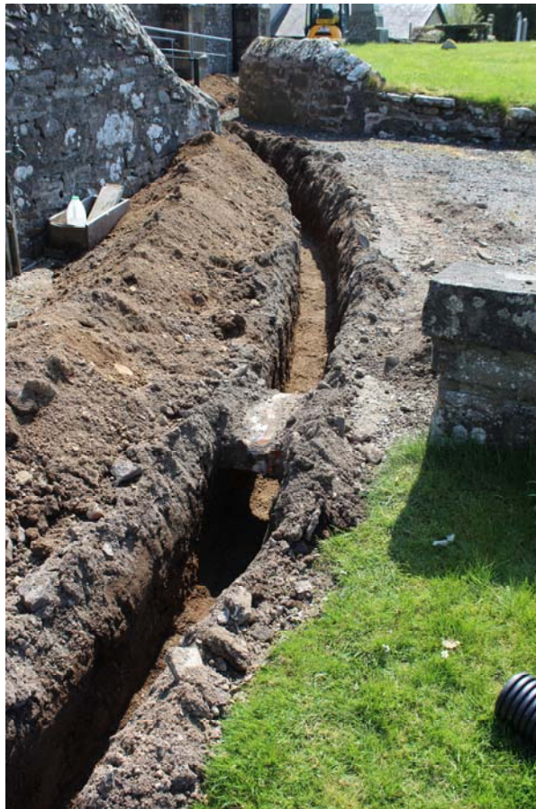
Plate 1: Cable track running adjacent to church.
