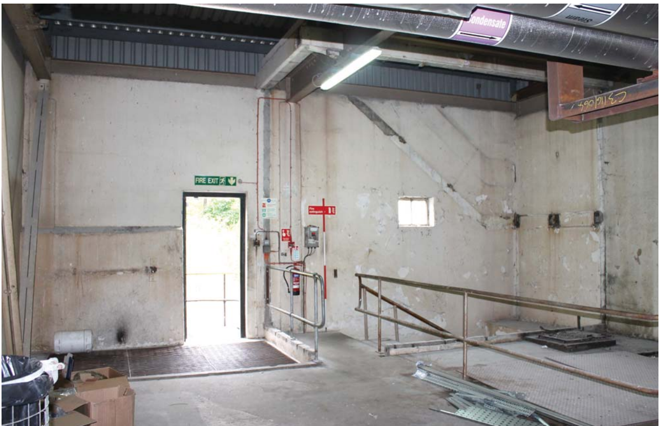
Plate 16: Hi Mac Building, general view of the attic level to the north-east side from the south-east
