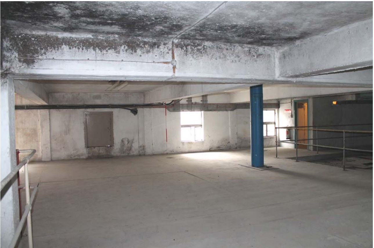
Plate 18: Hi Mac Building, general view of the empty second floor level to the south-west side, from the north-west
