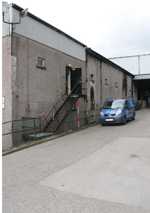
Plate 12: Hi Mac Building, general view of the north-west elevation from the north
