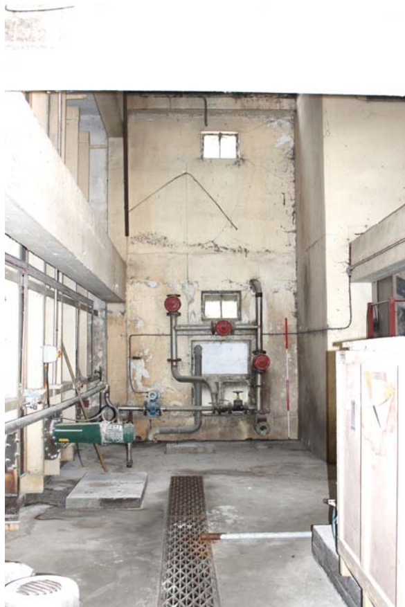
Plate 14: Hi Mac Building, general view of the interior to the north-east side from the south-east
