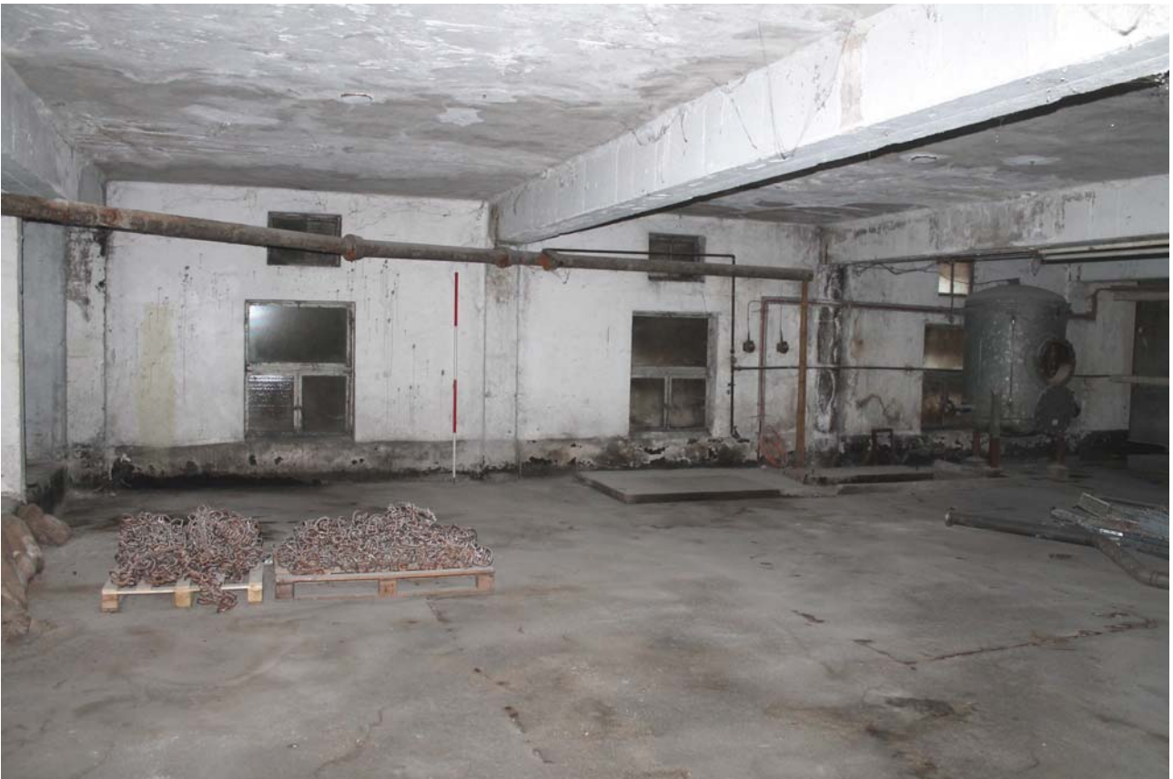
Plate 20: Hi Mac Building, general view of the empty first floor level to the south-west side, from the south
