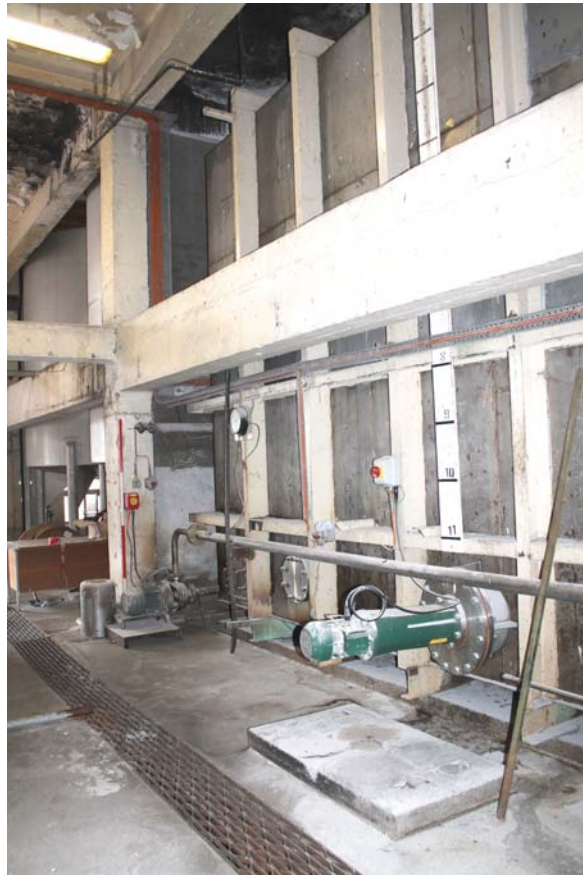
Plate 15: Hi Mac Building, general view of the interior to the north-east side from the north
