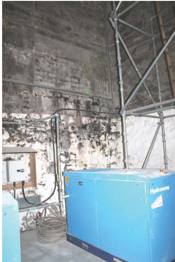
Plate 23: Malt Storage building, general view of the stone wall construction to the north corner of the building, from the south
