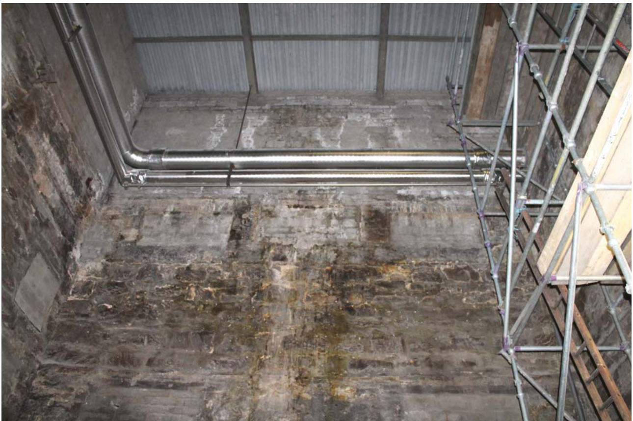
Plate 24: Malt Storage building, general view of the stone wall construction to the north corner of the building, from the south-west
