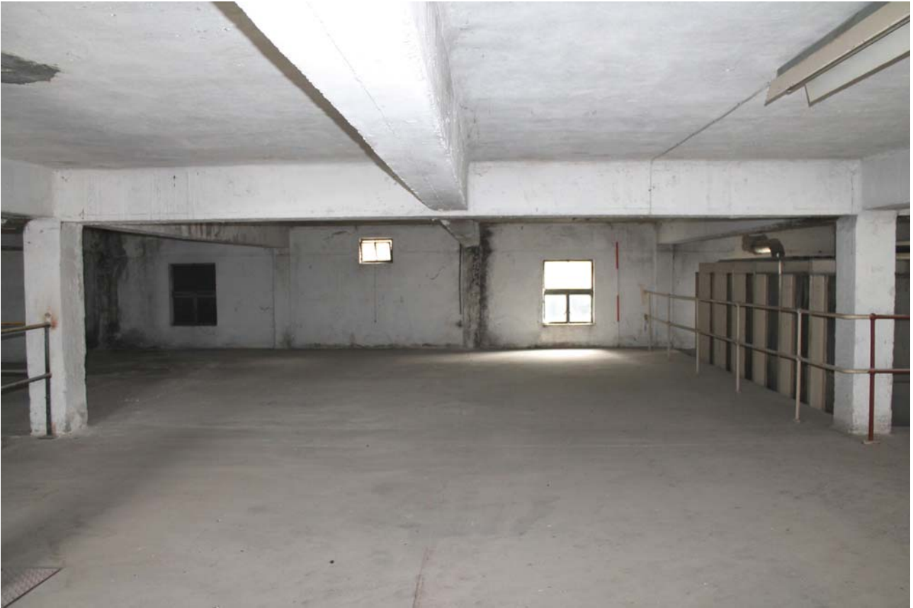
Plate 19: Hi Mac Building, general view of the empty first floor level to the south-west side, from the north-west
