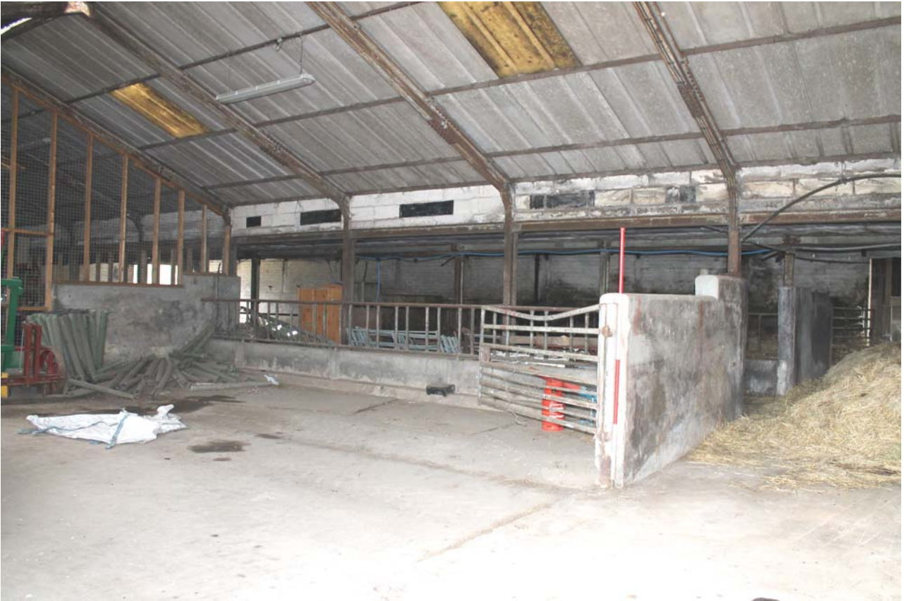
Plate 37: Farm Buildings, general view of the internal cow byre from the east
