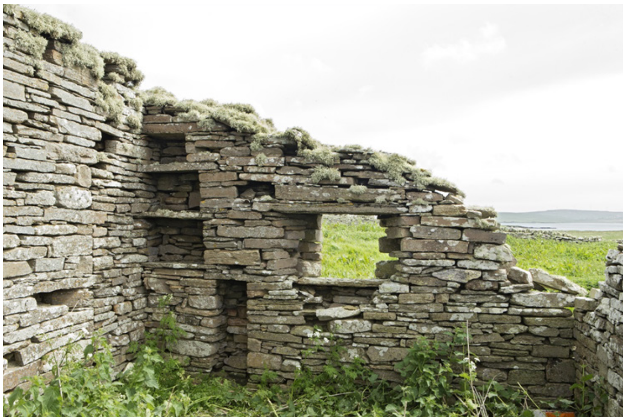
Illus 10. View from north of the stacked shelving, cheese-press and window in the south wall of the dairy. DP256478.
