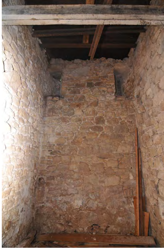
Plate 9 Interior north-facing elevation with blocked up slit vents near the wall head
