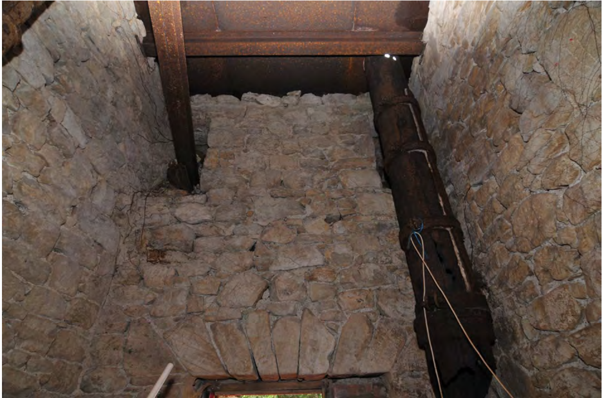
Plate 11 Interior south-facing elevation above the door with pipe work
