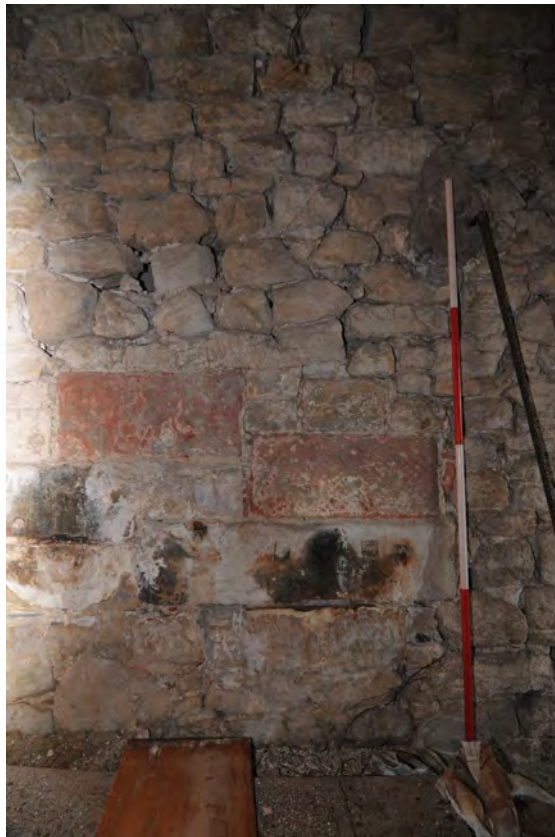
Plate 10 Interior east-facing elevation with oil stained masonry blocks
