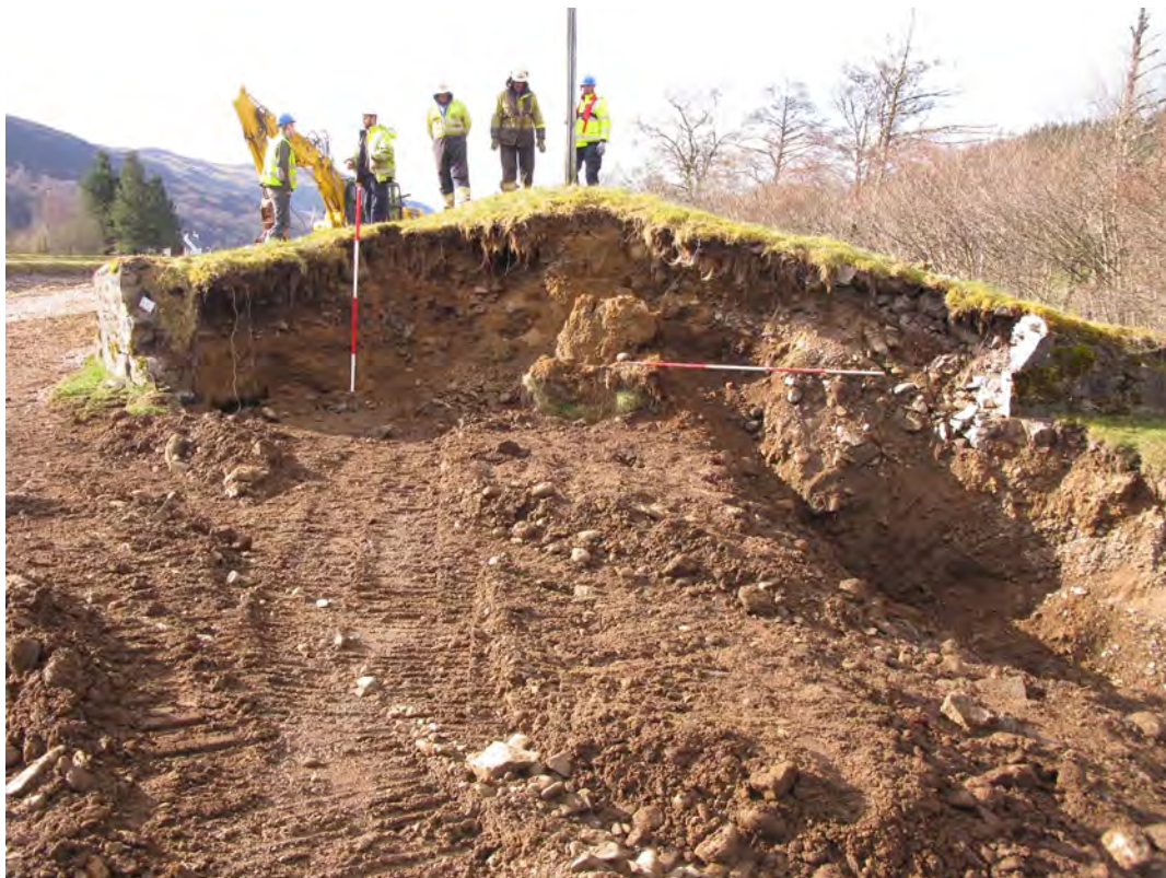
Fig. 4 Section through Canal bank at South-west end of weir showing remains of retaining wall
